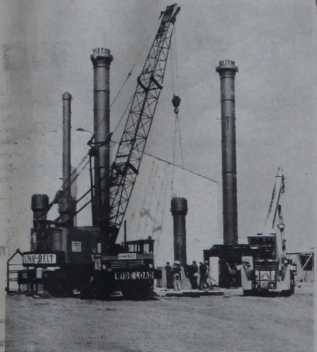
SHORT STACK —Using a crane hoist, workmen fit a short stack beside taller ones in the synthesis section of Western Ammonia's plant expansion. These stacks will help convert gases into anhydrous ammonia. In background is the new compressor building. This is one of five basic construction phases of the expansion, which is being erected by Universal Maintenance & Construction Co. of Houston.
