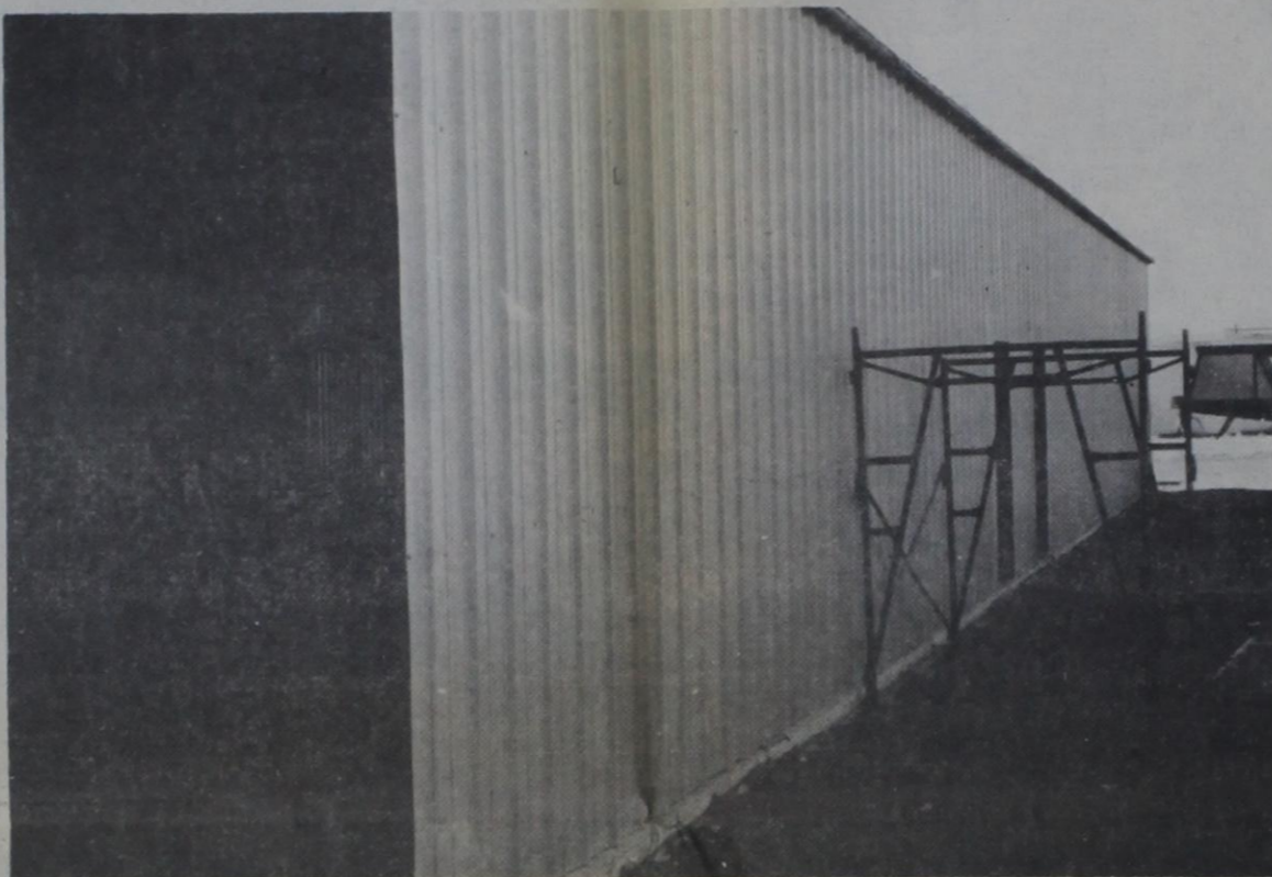
NEW ANNEX TO DIMMITT EQUIPMENT CO. ... Increases size of parts department and shop
