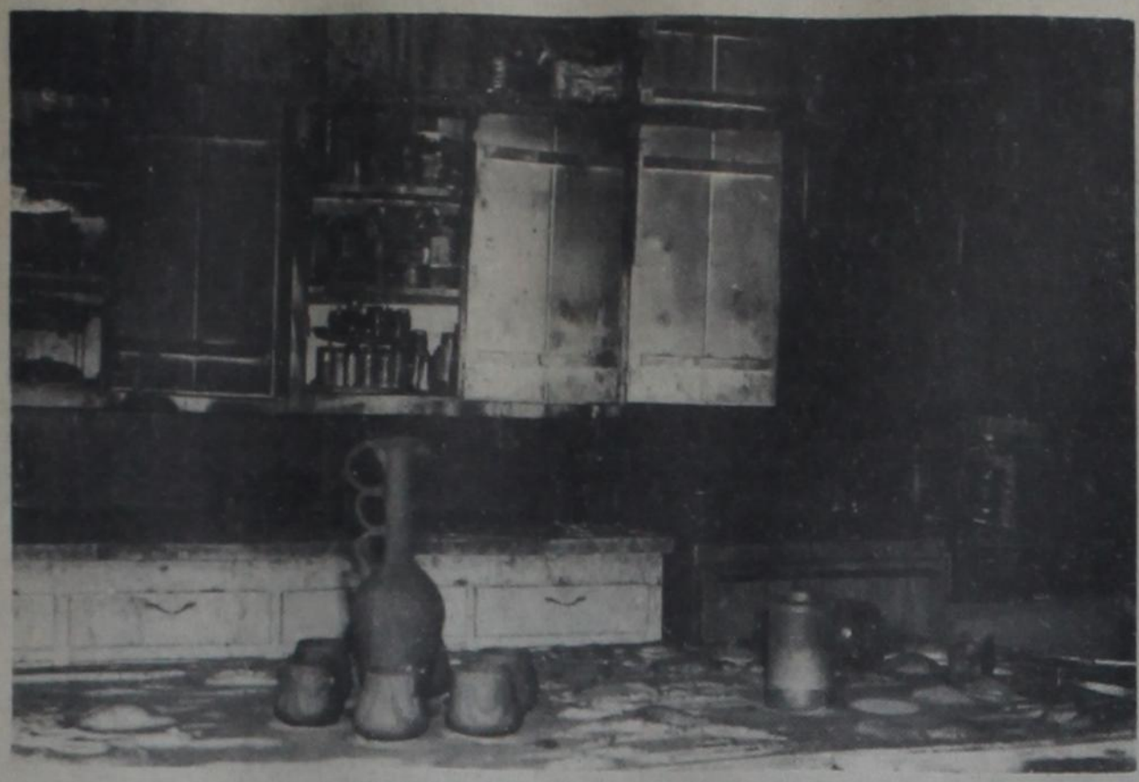
RUINED KITCHEN IN RONNIE IVY HOME. Christmas decorations were already up when fire struck
