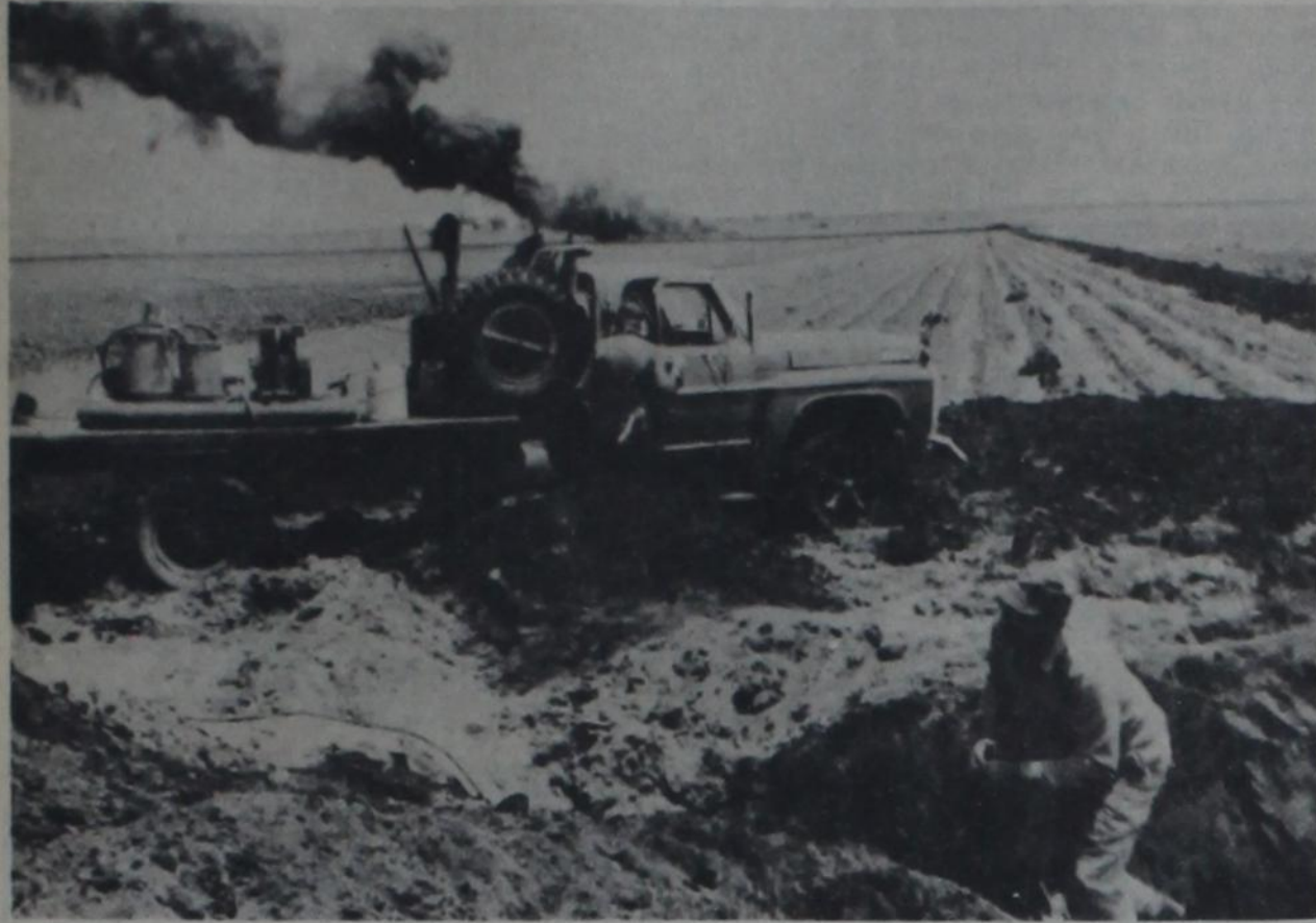
UNPLANNED GUSHER —Phillips Petroleum Co. workmen repair an oil-line break that sent thousands of gallons of crude oil gushing to the surface last Thursday on the farm of Harold Bob Bennett, seven miles southwest of Hart. In background, smoke billows from a pool of oil being burned off
