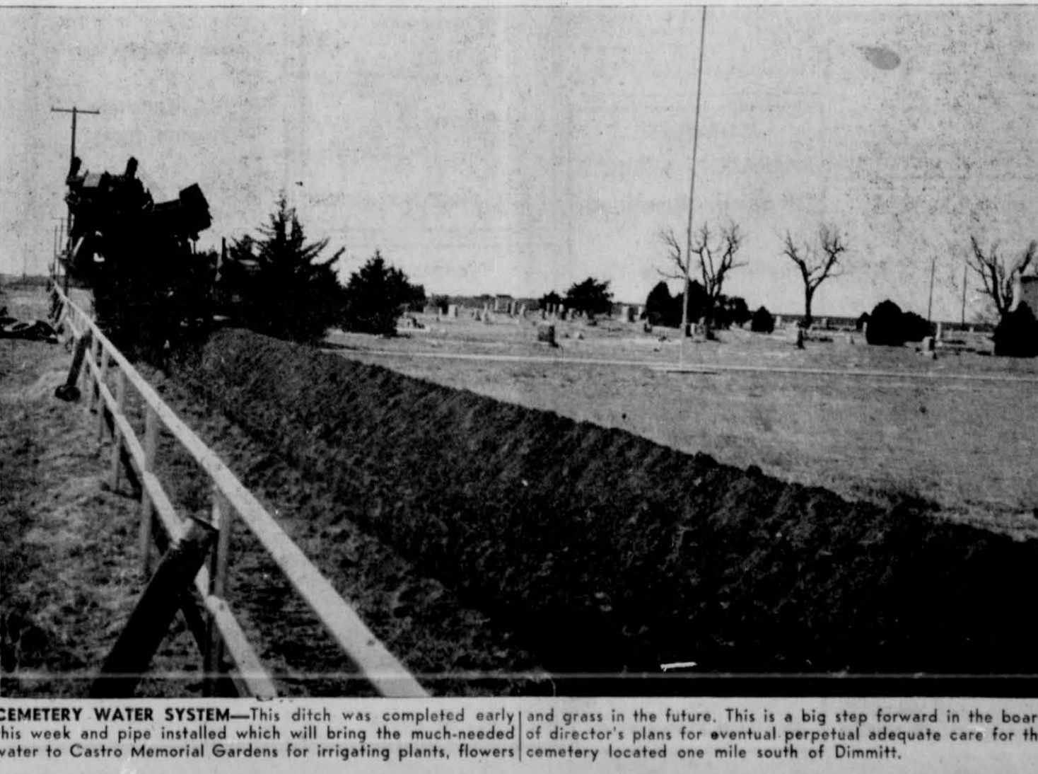
CEMETERY WATER SYSTEM—This ditch was completed early this week and pipe installed which will bring the much-needed water to Castro Memorial Gardens for irrigating plants, flowers and grass in the future. This is a big step forward in the board of director's plans for eventual perpetual adequate care for the cemetery located one mile south of Dimmitt.
