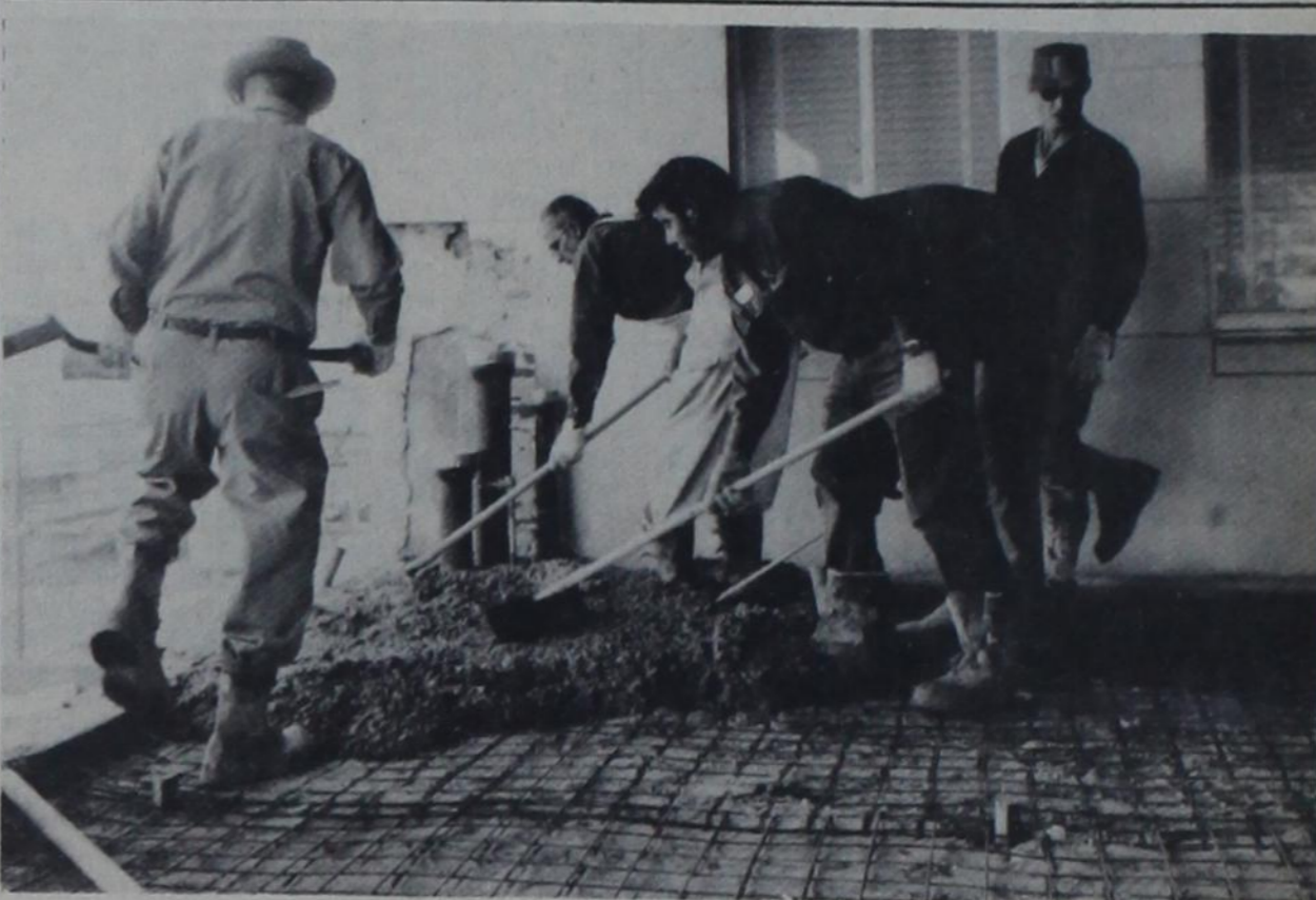
ONE FLOOR, COMING UP — Workers poured and smoothed out the first floor of the new courthouse annex last Wednesday to complete the basic structural concrete phase of the construction. The massive concrete skeleton for the addition now shows what the new dimensions of the courthouse will be when the project is completed. (Photo by Darla Kay)
