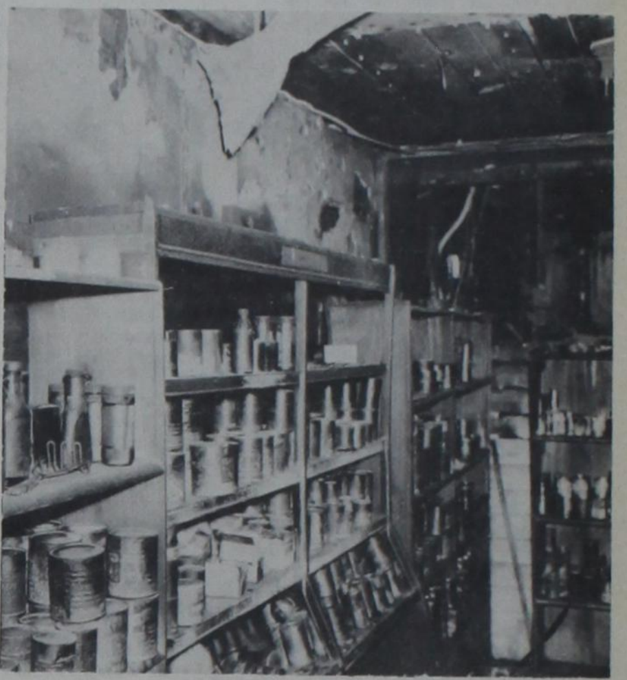
DAMAGE WAS HEAVY throughout the building in last week's fire at Hacker's Grocery, but some of the merchandise was salvaged. The fire was discovered by Whitfield Truck Line drivers passing by, who reported it and notified Mrs. Hacker's family. A three-layer ceiling hindered firemen's efforts.
