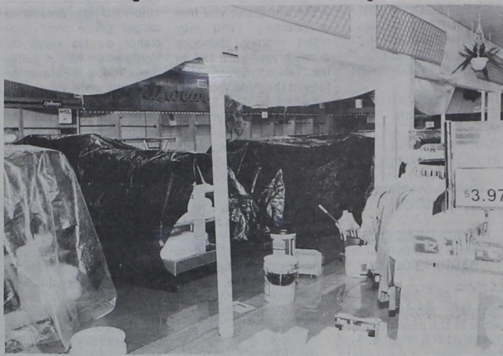
ANOTHER RESULT of the recent heavy rains in the county has been water damage at the C.R. Anthony store in Dimmitt, which was in the process of getting a new roof installed. With the old roofing materials stripped off and the new not installed, a lot of water
