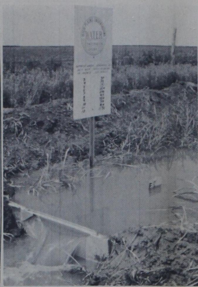
A WEIR INSTALLATION located on the Deaf Smith, Castro county line. Notice the water is running 10" deep through the discharge slot in the weir. Comparing the 10" discharge to the large sign, one can easily see 719 gallons per minute is passing through the weir. This water was escaping from an irrigation farm. Can this waste be ignored?
