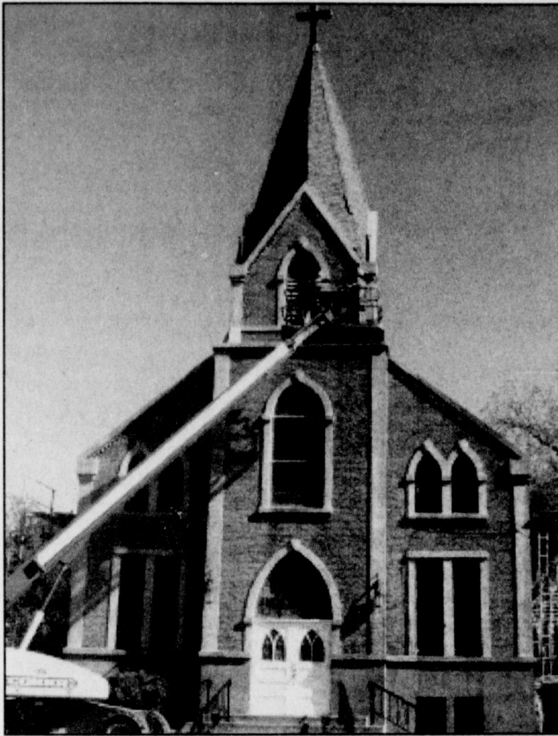
A TALL ORDER was recently filled by Jimmy Ripley and John Wilson of Straight Line Construction as they rose to the occasion to replace the roofing of St. John's Lutheran Church. (photo by Jean Boles)
