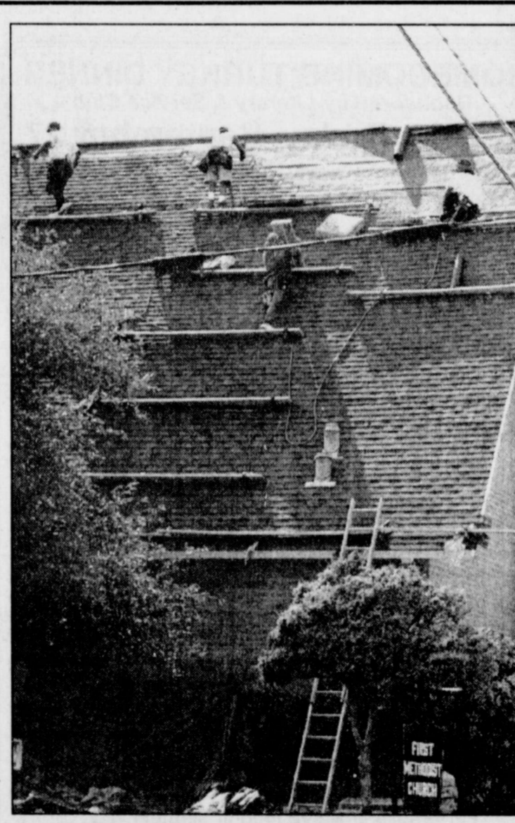
TEDIOUS TIPTOE WORK was the order of the day as these roofers finish work on the steep slope of the First United Methodist Church. The church will dedicate a historic site marker this Sunday, September 22.
