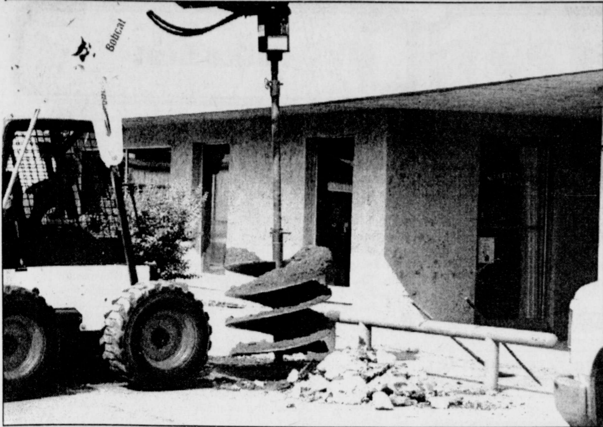
ALDERMAN-CAVE has begun work to relocate the time and temperature sign which was ordered by the Texas Department of Transportation to be removed from its location of more than 18 years. The sign, which is considered a landmark in Winters, will be moved a few feet closer to the building at a substantial cost to Alderman-Cave.
