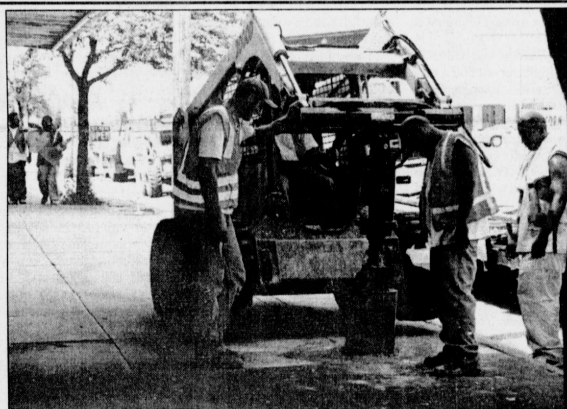
CONSTRUCTION WORKERS with Texas Commercial Fence, Inc., of Burnet, Texas, subcontracted by Texas Department of Transportation, drill into the sidewalk at the corner of Main and West Dale in preparation for moving another state traffic sign. The project is part of a state-wide mandate to improve safety.
