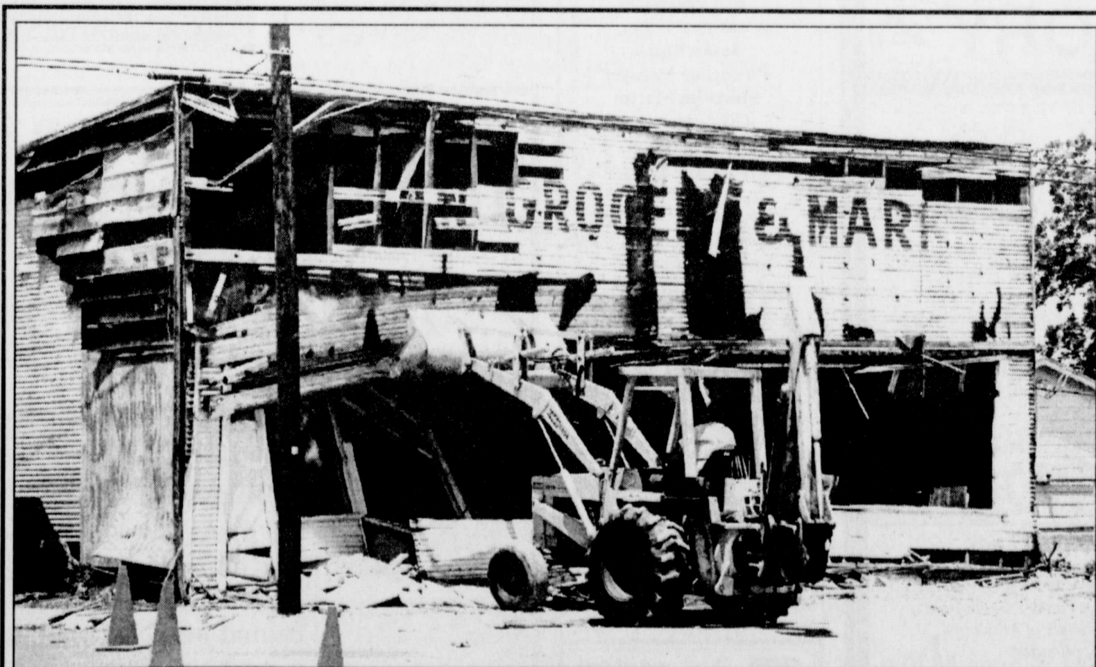
AND THE WALLS CAME TUMBLING DOWN, thanks to Charles Grenwelge, Street Superintendent, operating the front end loader. The old building, possibly built in the 1930's at the corner of East Dale and Grant Streets, was demolished last week by city employees as part of an ongoing effort to improve the city's appearance. The structure was once home to Bratton Grocery, Huffman Grocery, Shirley & Jackie Howard's used furniture and refinishing store, a western wear store owned by Jeryl & Caroline Priddy, and a secondhand store operated by Ray Hale.
