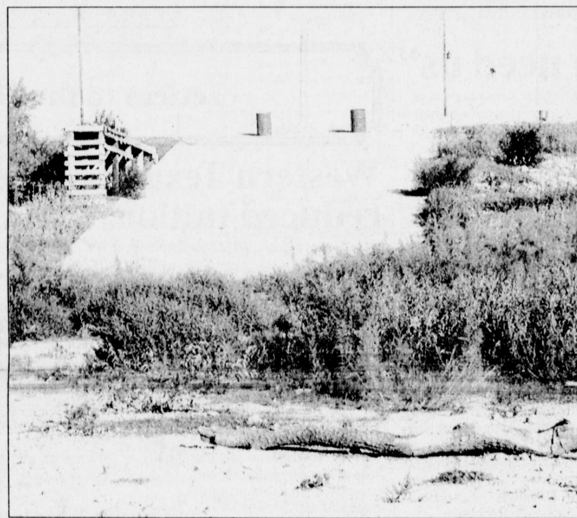
ONE VERY DRY DOCK is the case at Elm Creek Reservoir where the water level continues to drop. The City of Winters is hoping to utilize the pipeline being brought from Ivie Reservoir to Abilene. The pipeline will run within about four miles of Winters' existing water lines and is hoped to be available by late next summer or early fall.
