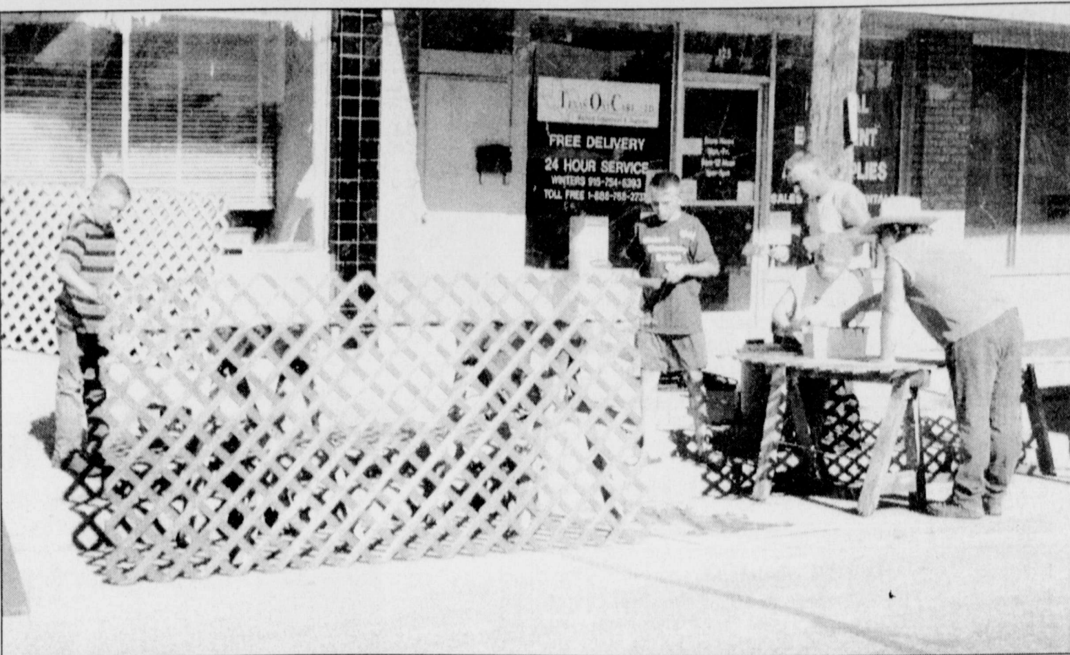
GIVING SOMETHING BACK TO THE COMMUNITY are these Winters 4-Hers and their fathers who along with other club members and leaders have been painting, cleaning, and repairing this storefront at 121 N. Main. In an effort to help beautify downtown Winters the club "adopted" this location and plans to exhibit photography projects in the windows in mid-September. Working last weekend were (l-r) Colby Pritchard, Cody Pritchard, Johnny Pritchard, Trenton Grohman, and Freddie Grohman.
