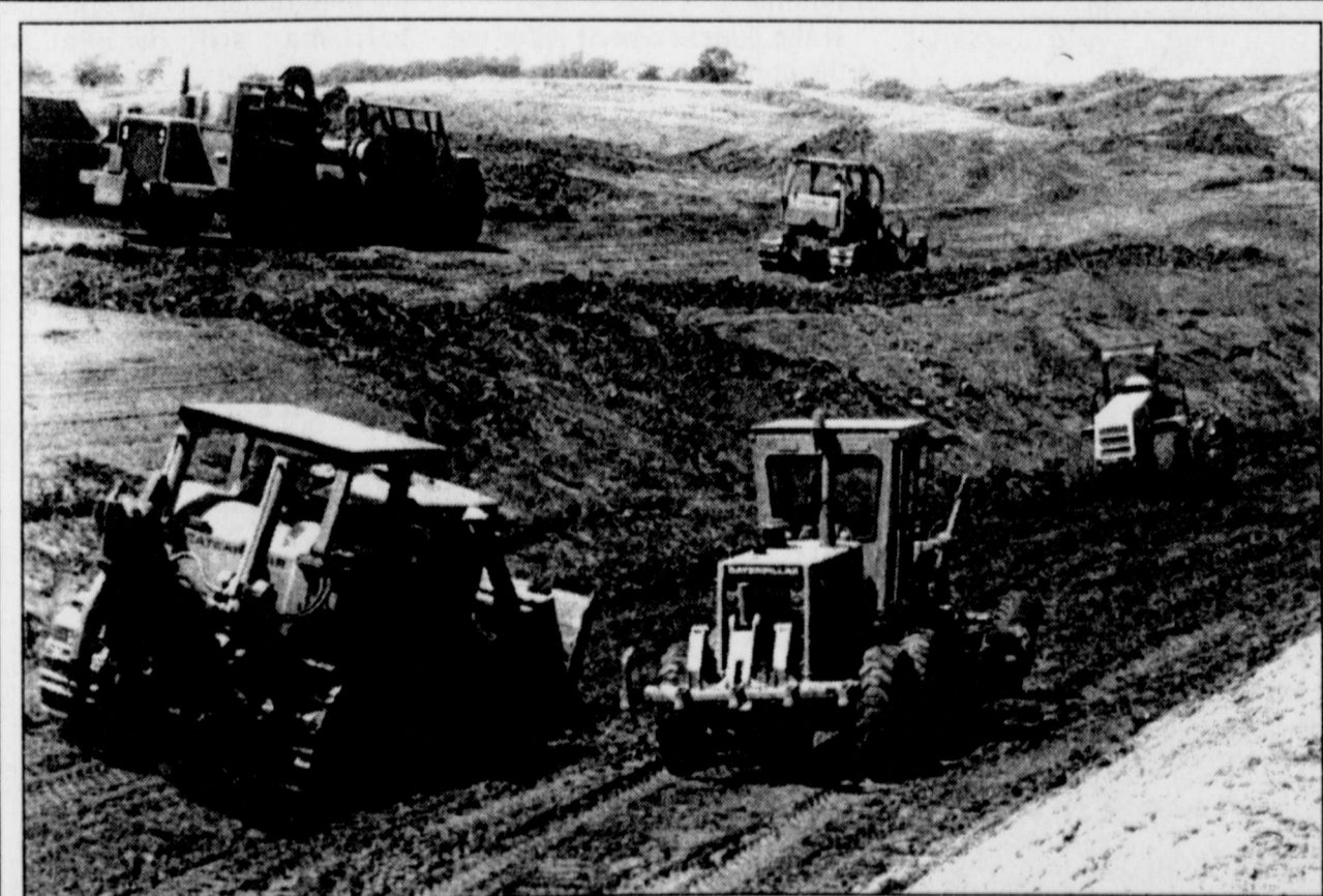
AFTER HITTING WATER-BEARING GRAVEL at the core grade level of a flood retention dam on the Galatian Ranch near Winters, the contractor removed the gravel and, in the photo above, is working to pack and dry out the soil. Once that is completed, the lower area will be backfilled to form the base of the dam.
