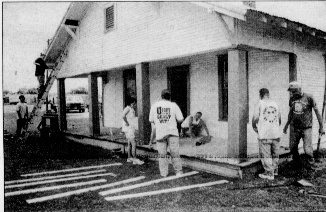
A GROUP EFFORT FROM (l-r) Sergio Rangel (on ladder), Tina Perrie, Andrew Medina, Marci Paschal, Larry Herring & Bryan Webb work on several areas of this home under the direction of house captain, Lanny Bahlman.
