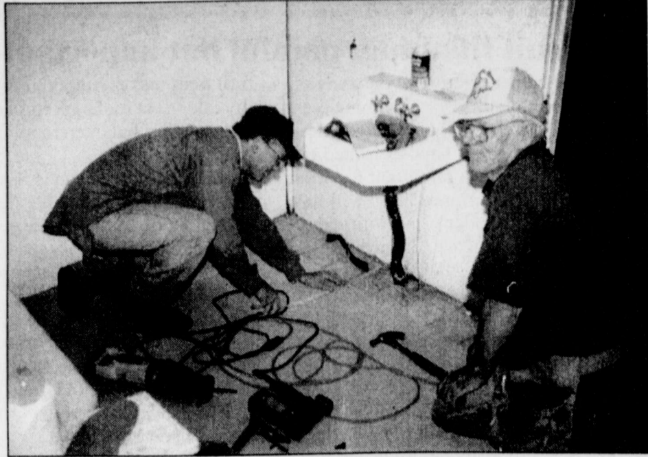
NEW FLOORING IS INSTALLED by Craig Gehrels (left) and Lee Harrison, part of Bob Lindley's house crew.
