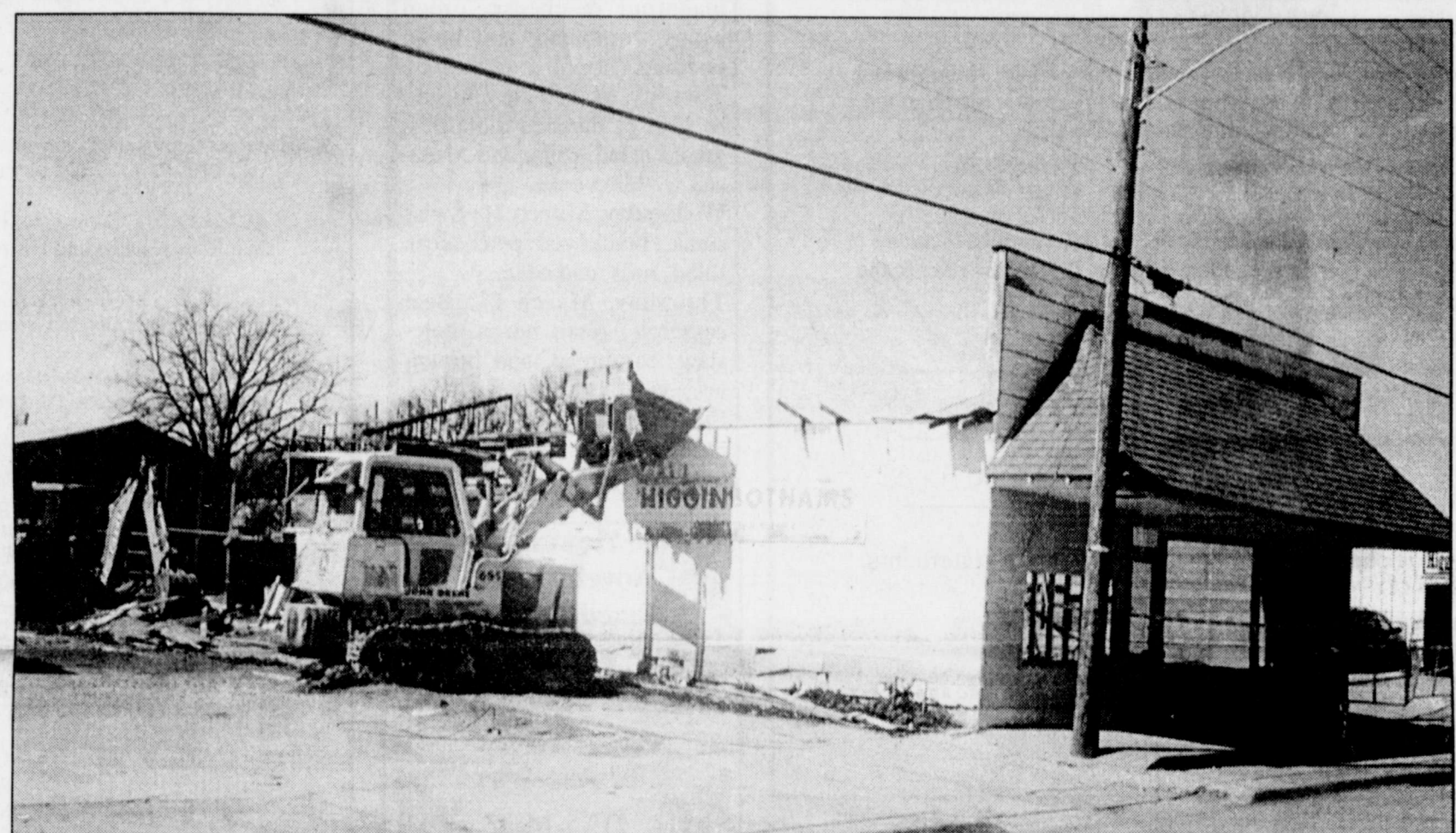
MAKING WAY FOR PROGRESS is the plan for Higginbotham's at 205 N. Main as workers demolish the old building on the south side of the property. Although the exact age of the building is unknown, some local citizens "guess-timate" that it was constructed in the late 1920's or early '30's. Local manager Dawn Green said the company is "very excited" about the new look which will be landscaped and utilized for increased parking and easier access for customers. Higginbotham's offers a wide variety of merchandise and services including lawn and garden supplies, a full lumber yard, hardware including Dewalt tools, Best paint, and unique gift items.
