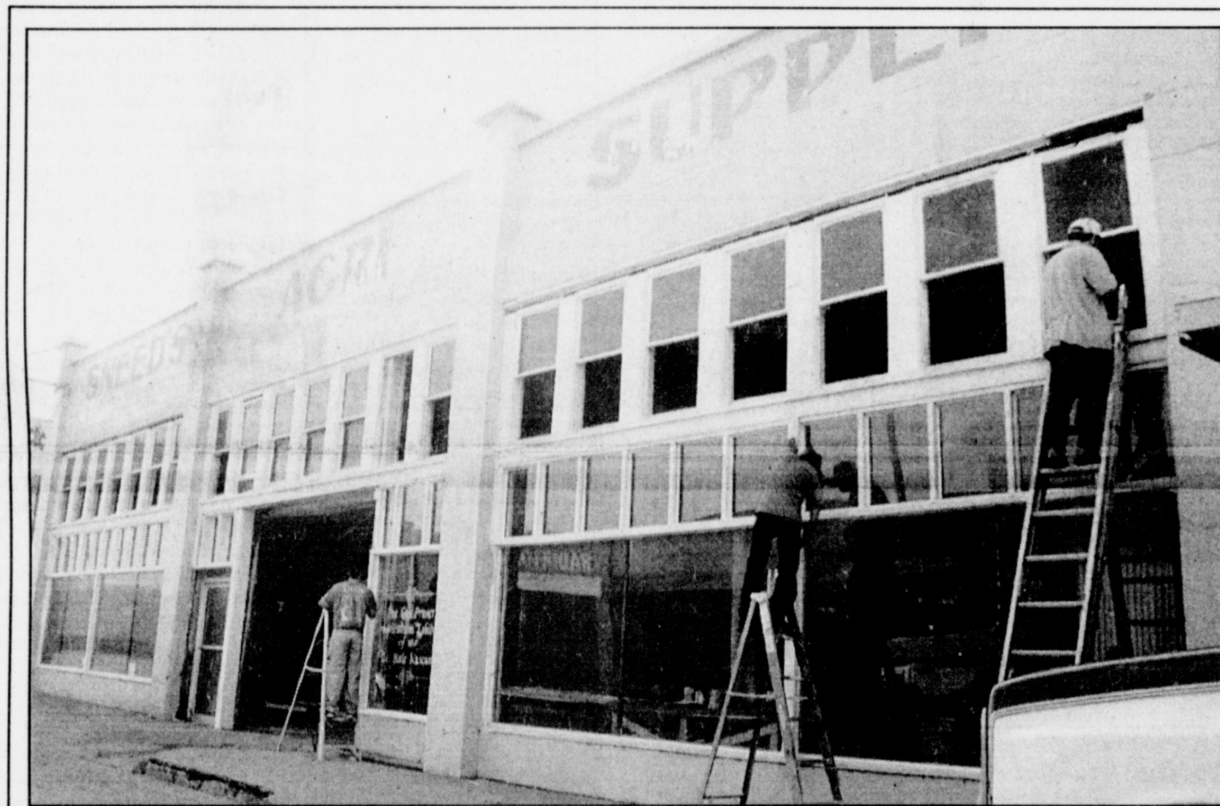
THE GUS PRUSER AGRICULTURAL EXHIBIT of the Z. I. Hale Museum is undergoing construction in the old building at 219 West Dale. Named for Winters pioneer Gustav Adolph Pruser, the exhibit will house antique tractors, a 1905 horse-drawn hearse, a covered wagon, and other agricultural items. A work day is set for Nov. 15, beginning at 9 a.m.
