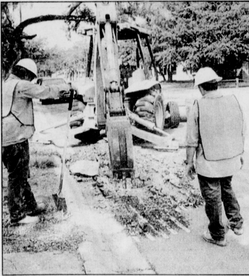
DIGGING FOR GAS LINES has been underway for several days in various parts of Winters. The Texas Railroad Commission has ordered that all Poly I pipe, which was installed in 1970, be replaced throughout the state.
