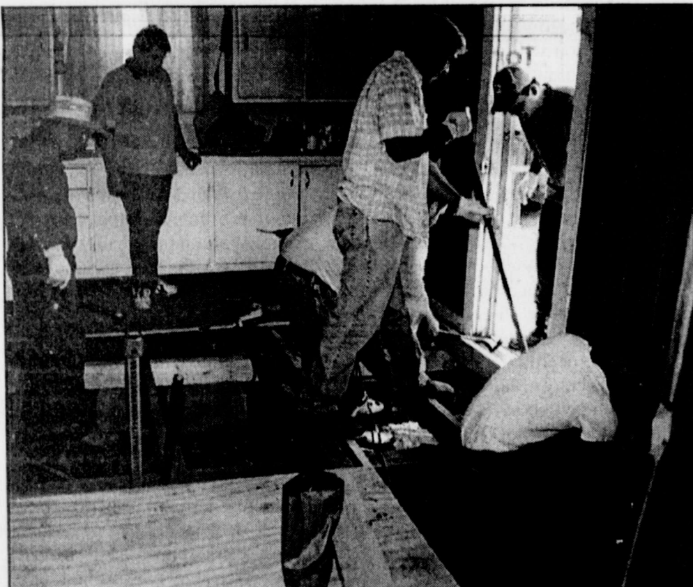
REPLACING AN ENTIRE KITCHEN FLOOR are volunteers for house captain Blas Lugo.
