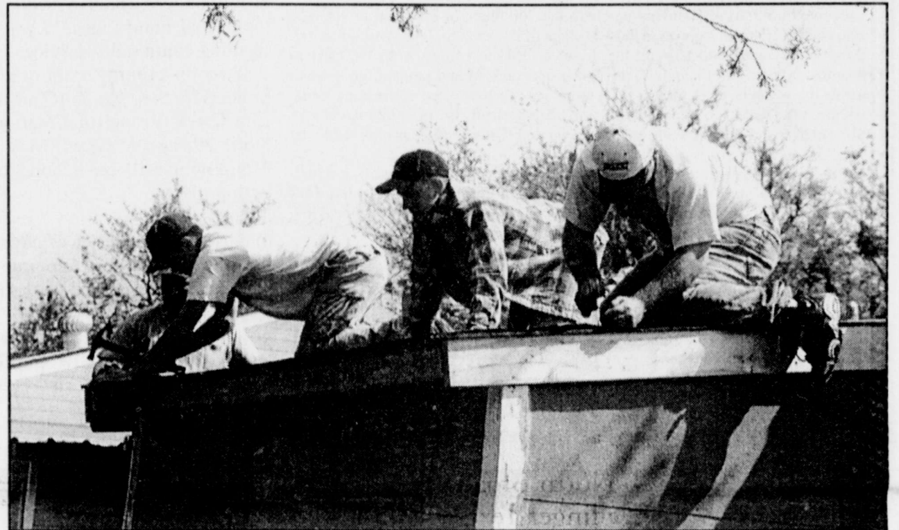
PUTTING ON A NEW ROOF at Phil Colburn's site are (l-r) Johnny Bob Pritchard, Shane Colburn, Guy Slimp and Michael Mostad.
