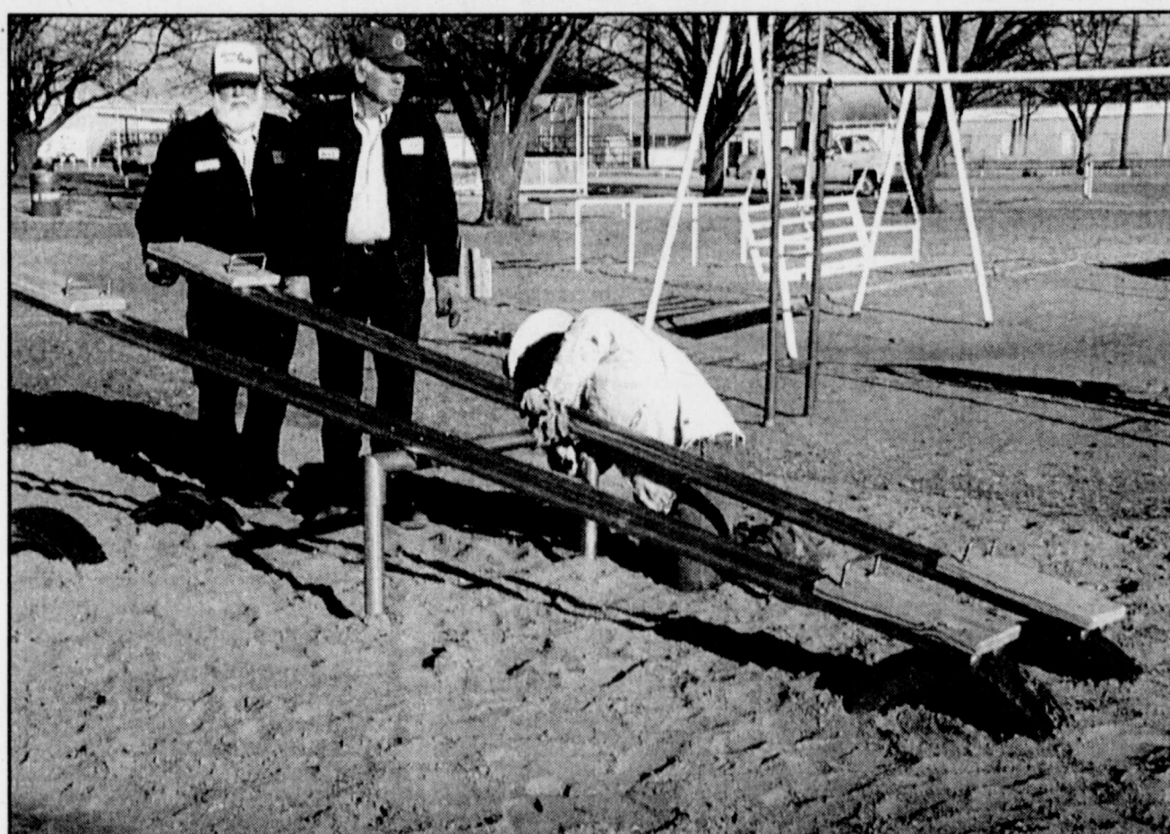
CITY OF WINTERS EMPLOYEES (l-r) Pete Gray and Jack Burns inspect Freddie Grohman's work as he puts finishing touches on the new four seated seesaw recently installed on the playground at Winters City Park. The seesaw was purchased by the Lutheran Brotherhood and Women's Service League organizations and installed by the city. This is the second piece of new equipment added to the playground in the last year. In addition, the city is repairing and replacing other worn out equipment, which has been on the playground for several years, filling holes, and adding sand to the playground area. The city park playground improvement campaign has been an ongoing project of the Women's Service League for the past four years.
