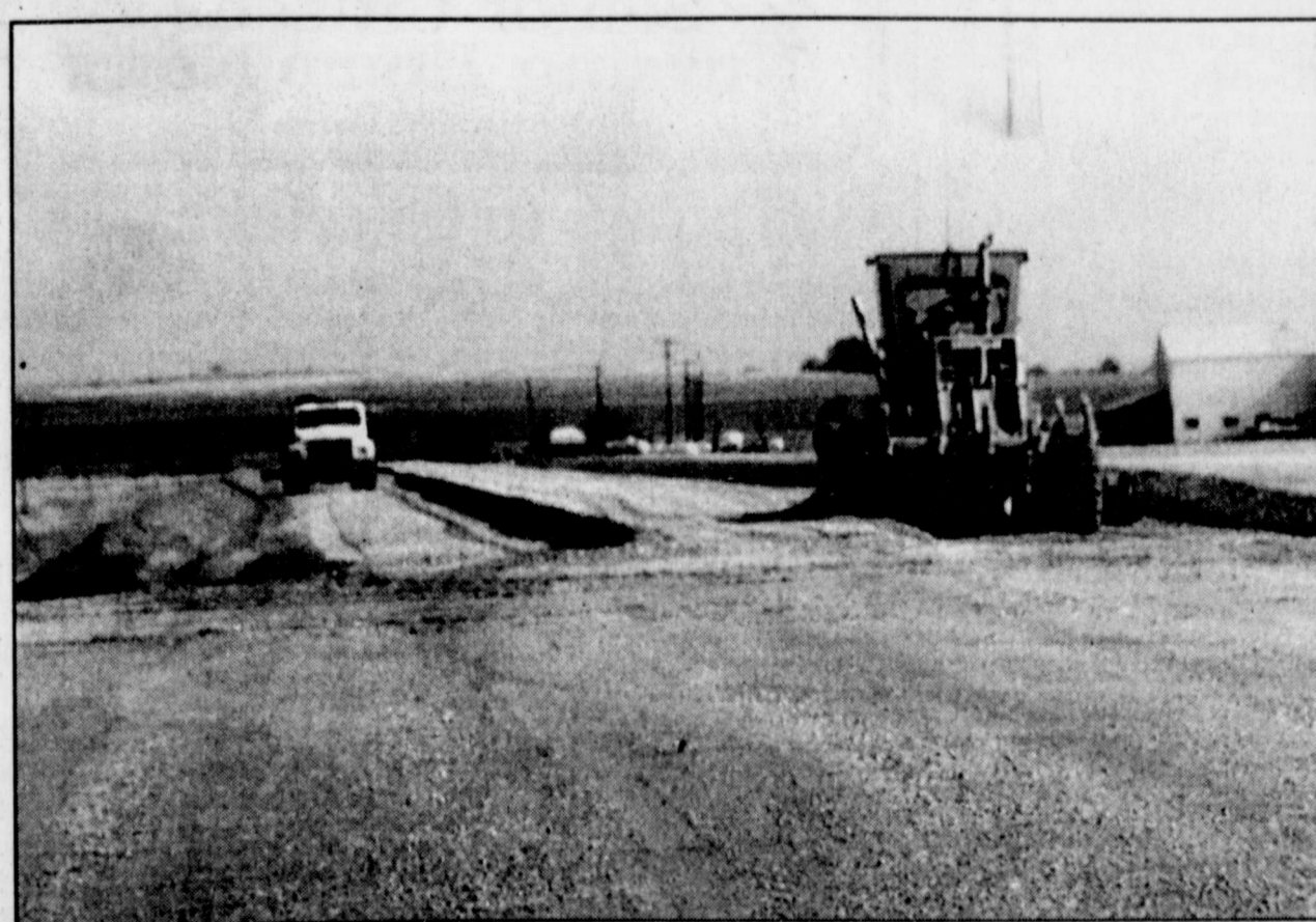
AIRPORT CONSTRUCTION continues as six inches of flexbase is being covered by workers from Prater Equipment Company of Comanche. According to City Manger Aref Hassan, work is still on schedule for completion at the end of September.
