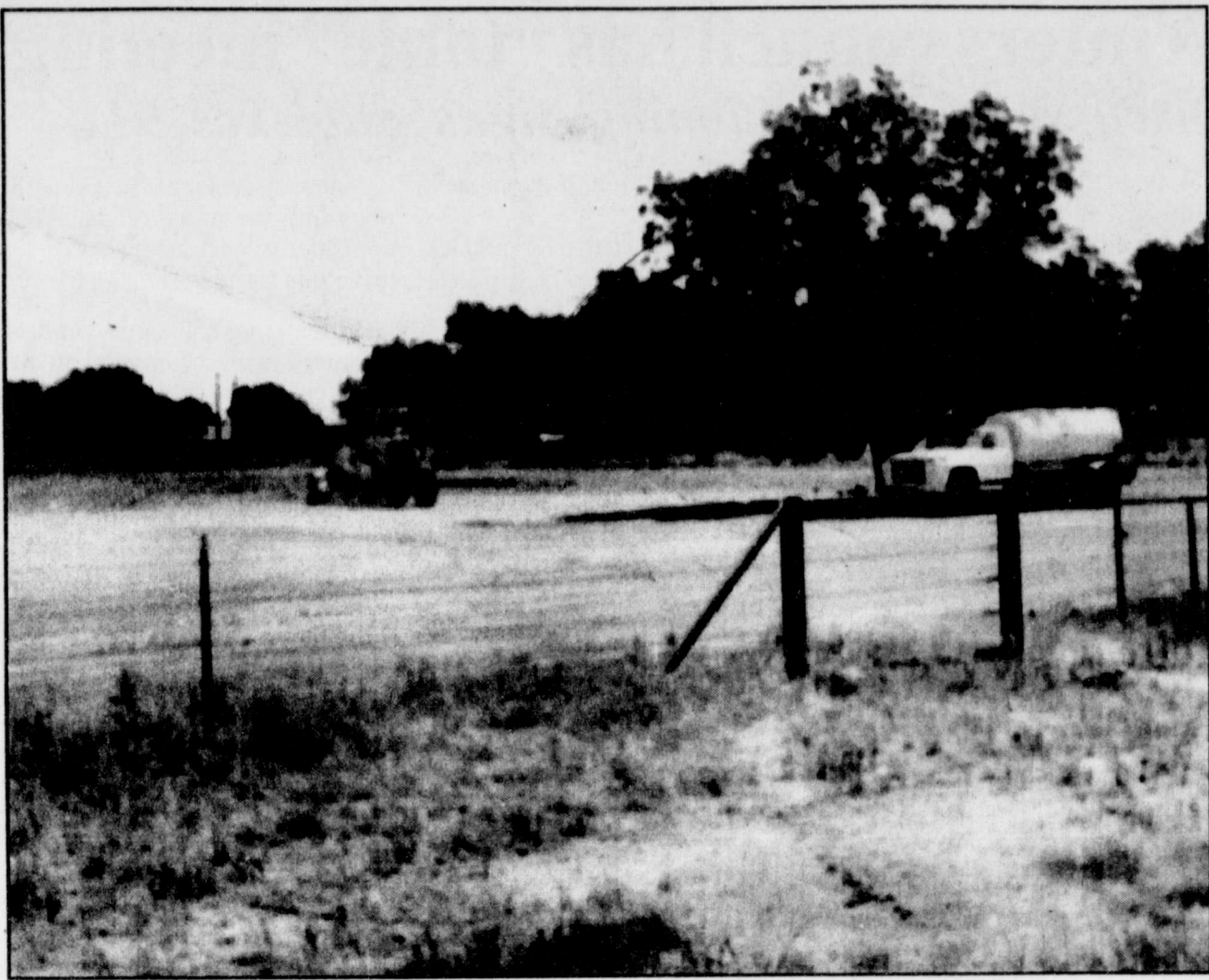
HOUSING DUPLEX CONSTRUCTION is now underway at the north end of town on Highway 83. Plans are to build 25 two and three -bedroom duplexes to help ease the housing shortage in Winters. The $3 million project, which has been in the planning stages since late 1997, is under the guidance of the Housing Finance Corporation of Winters. Duplexes will rent for around $400 to $500 per month.
