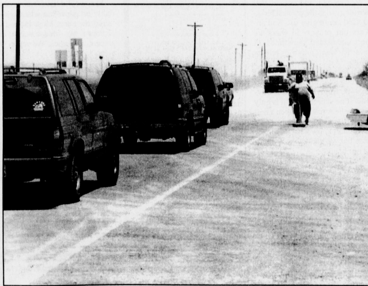
POE'S CORNER TRAFFIC CONGESTION has been a regular happening as road construction continues on Highway 153 east and west of Winters. The 2.6 million dollar Texas Department of Transportation project was started in October, 1998, and should be completed by September, 1999.
