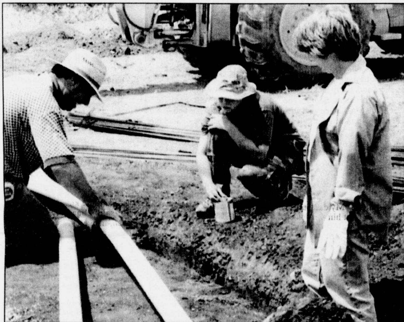
NEW CAR WASH CONSTRUCTION is underway at the corner of Main street and the Novice road. Building contractor Mike McDonald (left), connects pipe as Becky Airhart and son Jared watch. Becky and her husband Paul are the owners of the four-bay facility.
