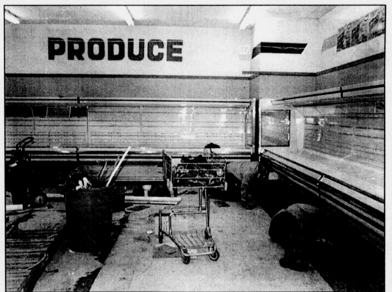
NO, THESE ARE NOT STORE EMPLOYEES looking for lost fruit, but construction workers hired by Lawrence Bros. to remodel the produce department. The store is currently undergoing several renovations.
