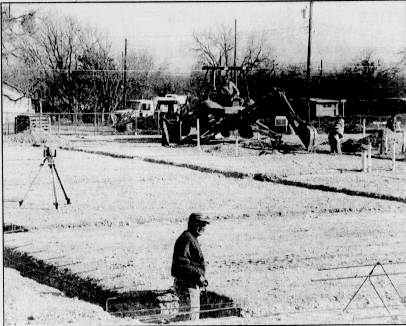
BARRON GUY of Guy's Dirt Contracting mans the backhoe while digging foundation work for the new junior high school. Construction schedule is on course thanks to recent sunny skies and good weather.
