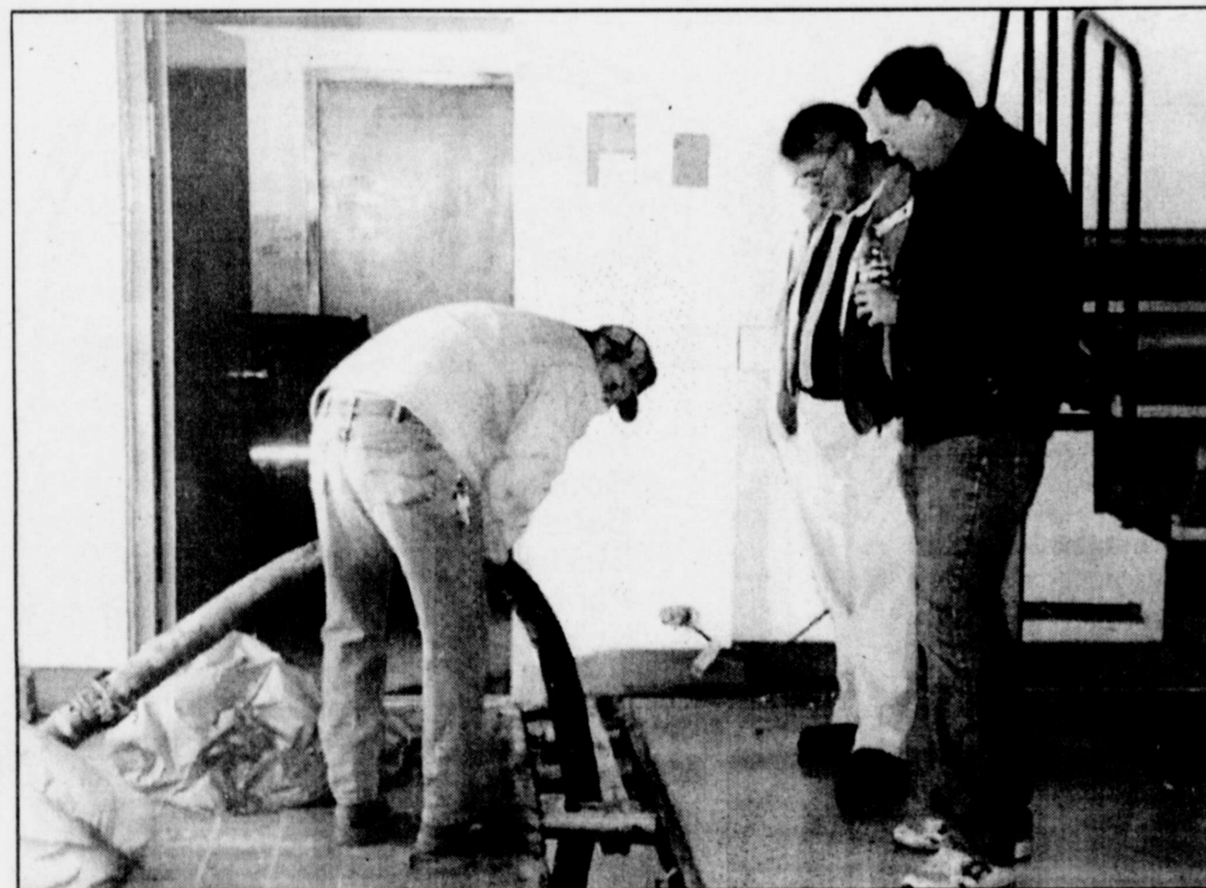
WATER, WATER EVERYWHERE and definitely not where it's needed. WISD superintendent Mike Harris, far right, and business manager Jimmy Butler watch as Mark Briley of the school maintenance department works to vacuum water from underneath the gym floor following a flooding incident. Cafeteria workers discovered the water about 5:30 a.m. on Dec. 16, which occurred when a pop-off valve on a boiler malfunctioned. On Friday, Harris said that approximately 15,000 gallons of water had been pumped from beneath the floor which had been refinished only last summer. Work continues to save the floor, but it is unknown at this time whether or not it will be usable for basketball, according to Harris.
