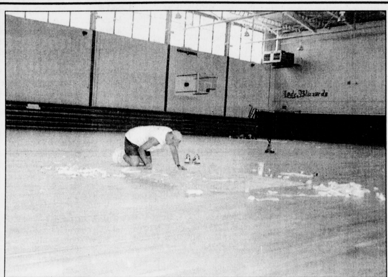
LYING DOWN ON THE JOB are employees of Hughes Services, Floor Resurfacing Division, of Lubbock as they repair the floor of the school gymnasium. Due to water damage, the floor had to be sanded down and resurfaced with new Blizzard and Lady Blizzard designs. The interior walls of the gym will also be painted to complement the new floor and logos.
