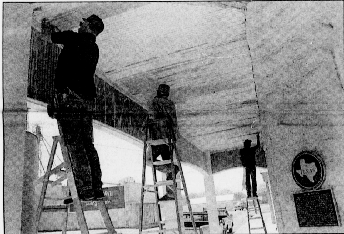
CONTINUING IMPROVEMENTS are being made at the Rock Hotel as evidenced by the scraping and painting done recently by (left to right) John Joeris, Wesley Wade and Donald Wade. The historic hotel has been undergoing extensive remodeling and has become a premiere landmark facility frequently used for various private and community functions.
