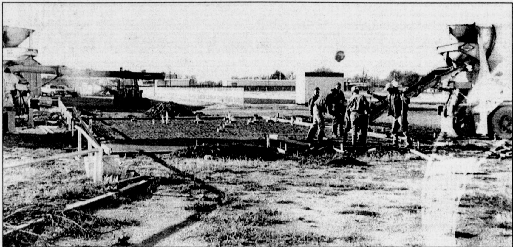
NEW CONCRETE FOUNDATION is ready to be poured for the track field facility which consists of a concession stand, restrooms and storage area located at the northeast corner of the track complex. Dale Montgomery, WISD maintenance supervisor, said he hopes to have the 1,800 square foot building completed by track season barring setbacks due to poor weather and delays in receiving construction materials.
