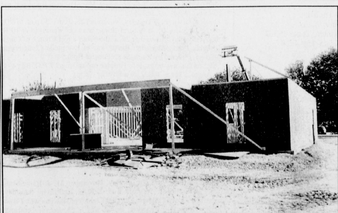
NEW SECURITY STATE BANK building is being constructed at 700 S. Main. The full-service bank will contain approximately 3,000 square feet. A crane hoisting a portion of the steel reinforced, pre-cast vault can be seen in background at far right.
