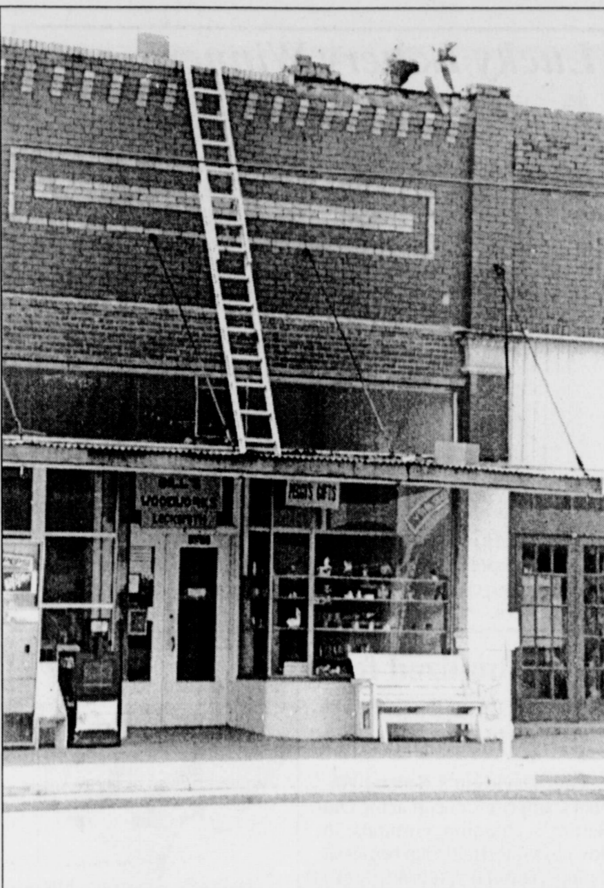
GETTING A "JUMP" ON CLEANUP DAY is Billy Ray of Bill's Woodworks and Locksmith on Main Street who went to great heights to improve his building. Saturday, August 9, has been designated as City-Wide Clean Up Day by the Winters Area Chamber of Commerce, and all business owners and residents are asked to make sure their properties are clean and attractive.
