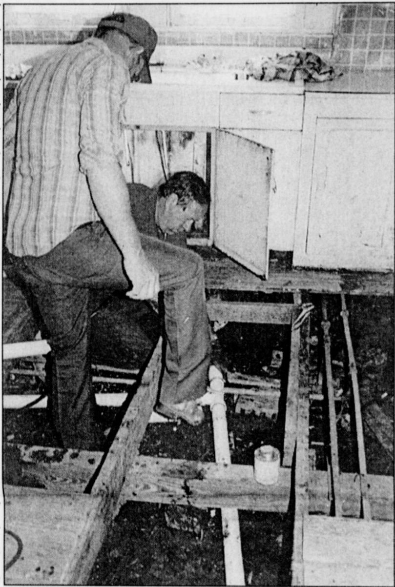
Paul Tharpe stands ready to lend a helping hand to Jerry Sartor, Sr., as they replaced broken plumbing and old flooring. Sartor is owner of Jerry Sartor Plumbing of Abilene and has donated his time and tools for the past three years for CIA.
