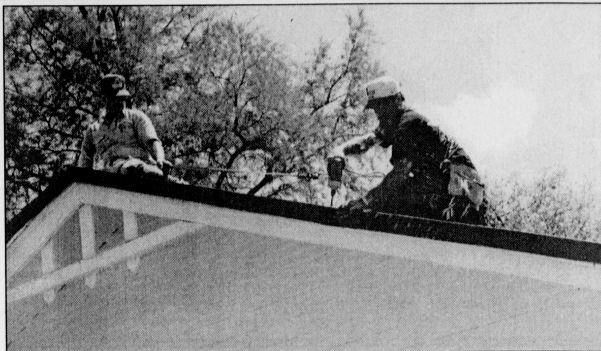
Robert Simpson provided some reassuring support to Chris Ozbirn as they worked high atop a roof being repaired.
