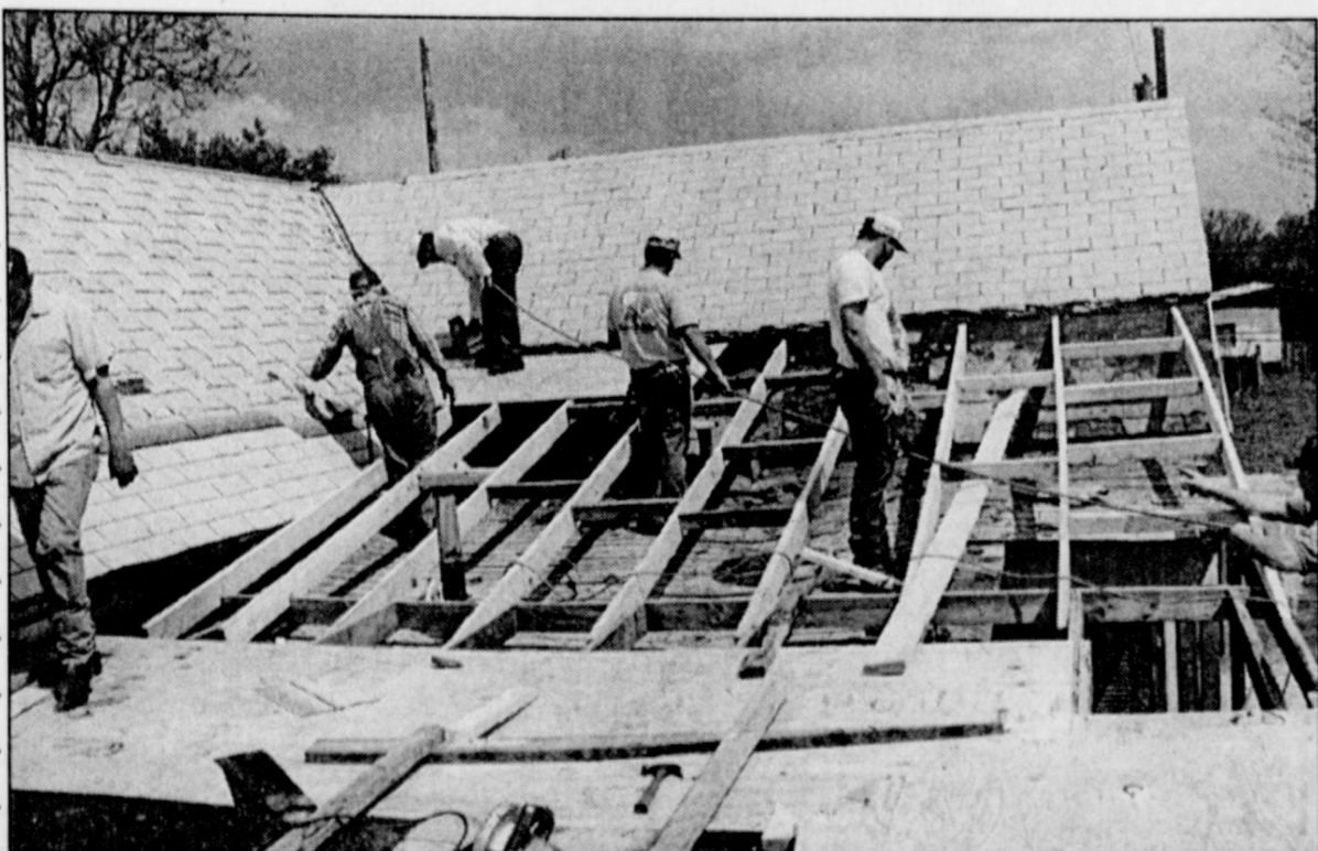
Builders didn't mind getting framed as they worked on a new roof.
