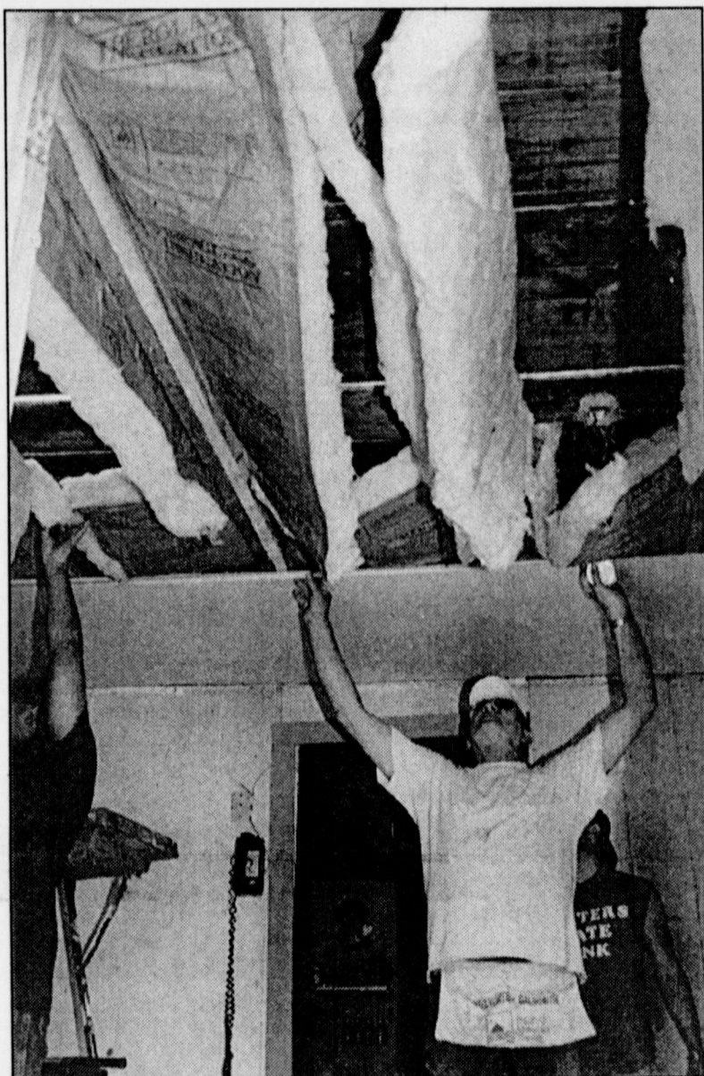
Charles Brewer and crew installed insulation and sheetrock for a new ceiling.
