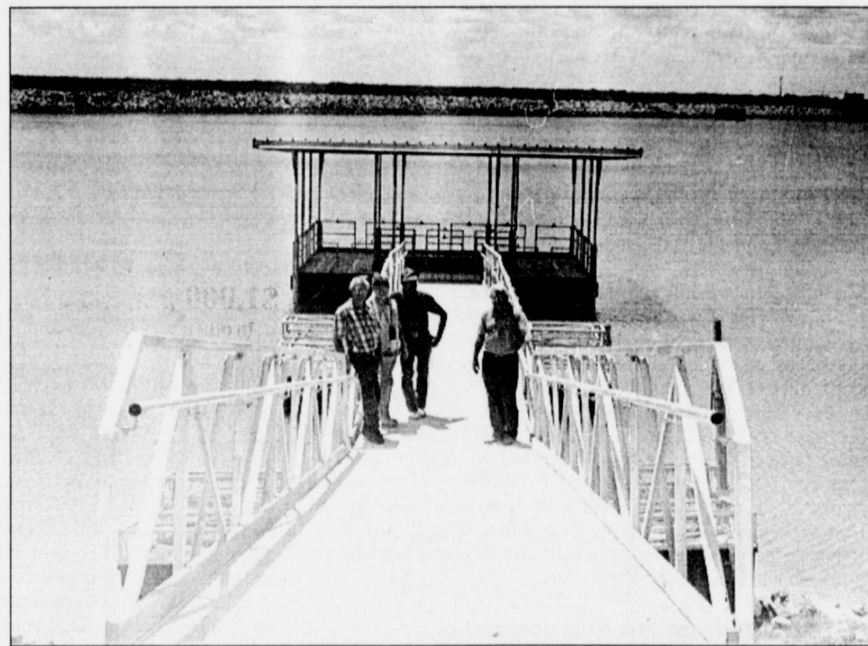
NEW FISHING PIER READY FOR USE at Elm Creek Reservoir—Top picture, several hundred pieces of metal and plastic, delivered August 15 by Galvan Foam of Missouri, await placement. Middle, Construction workers steady the first portion of the pier as it is lowered into position. Bottom, Mayor Dawson McGuffin, Lakekeepers Jean and Billy LaFair, and City Manager Aref Hassan go to inspect the finished product. Total construction took only five days.
