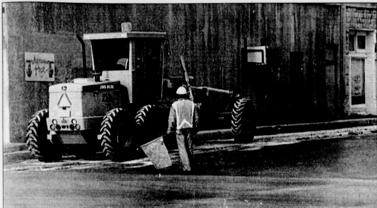
CUTTING DOWN THE BUMPS on West Dale Street at the intersection of U.S. 83, the Texas Department of Transportation is preparing the road surface for a hot mix pave in September. According to Carla Baize, TxDOT maintenance supervisor, West Dale Street will be paved from the U.S. 83 intersection to the city limit sign on Loop 438.
