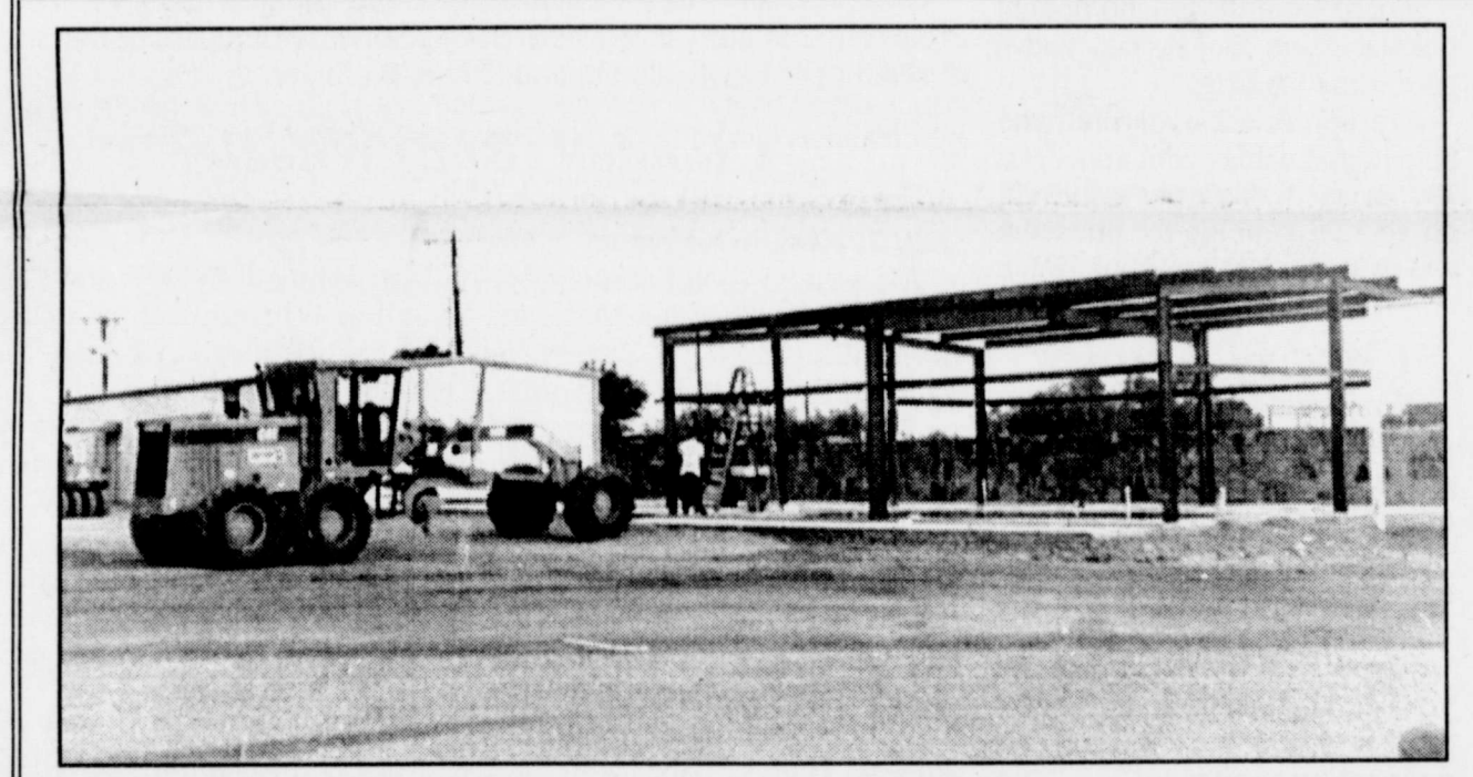
NEW CONCESSION STAND (right) at Blizzard field is taking shape as county workers smooth dirt to be gravel topped as part of the new construction and improvements in school property. The concession stand is a joint effort by the Blizzard Band Boosters and the Athletic Boosters. Volunteers are needed to help complete the project before the start of football season.
