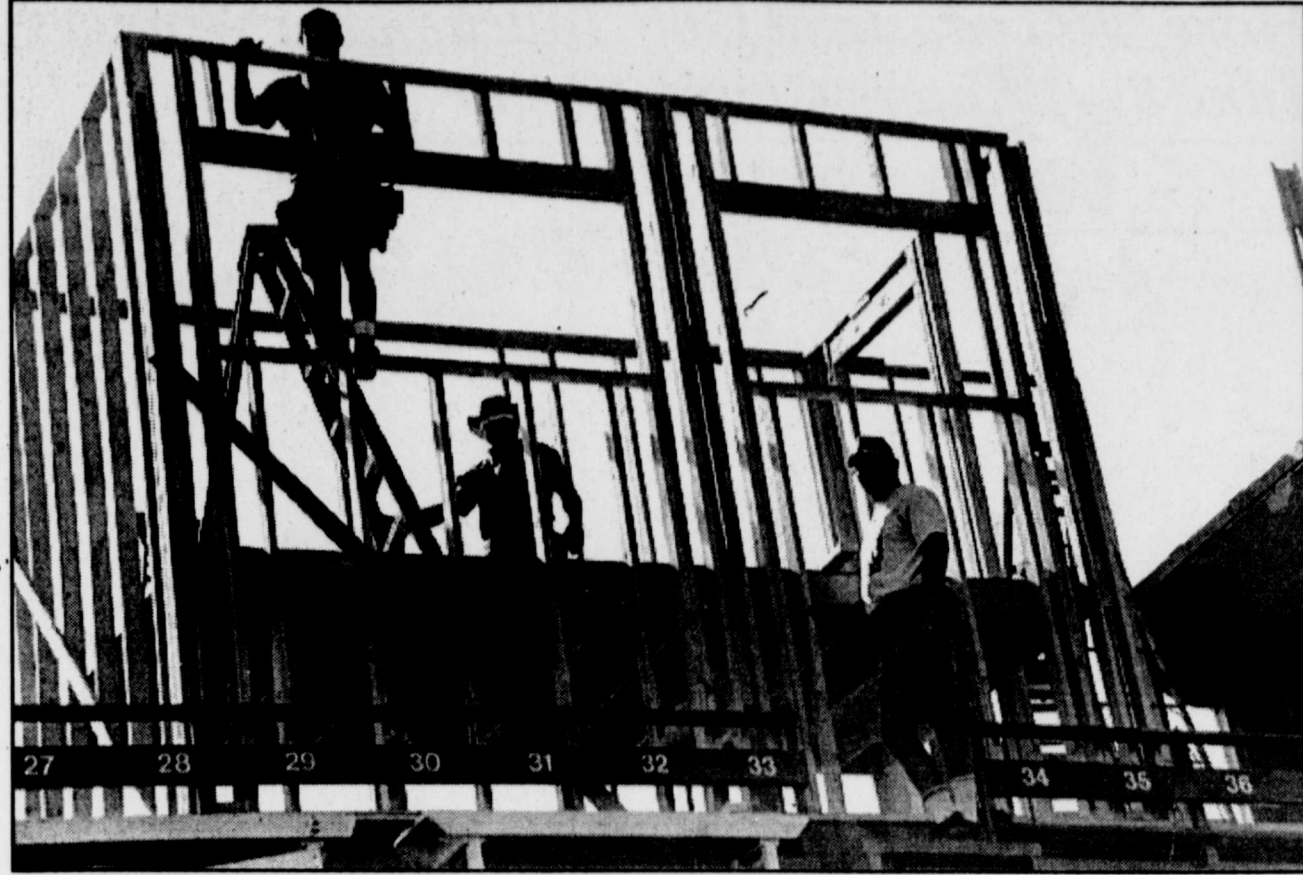
ERECTING A NEW PRESS BOX at Blizzard Field are Coach Chad Russell (on ladder), Johnny Merrill (center), and Coach Charles Murphy. According to Merrill, upon completion, the 50' long x 8' wide x 12' tall building will allow the film crew to complete their task much more easily than in the past. The bottom will be floored off to sit persons 4' higher. The north wall of the old press box will be removed, and the two will actually be joined. As a final touch, new front and back windows and siding will be installed. Approximate cost for these renovations is $2,500.
