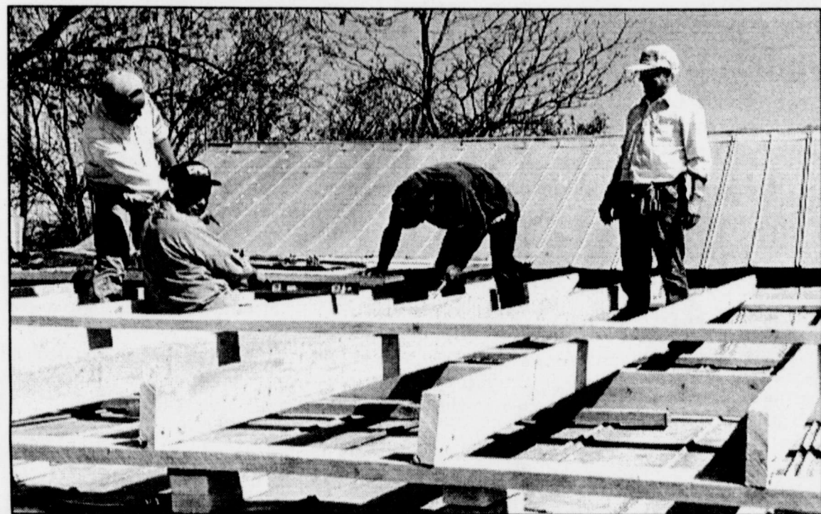
Mike Ramon, Rene' Cortez, George Mendoza and Nelan Bahlman assemble rafters for a new roof.
