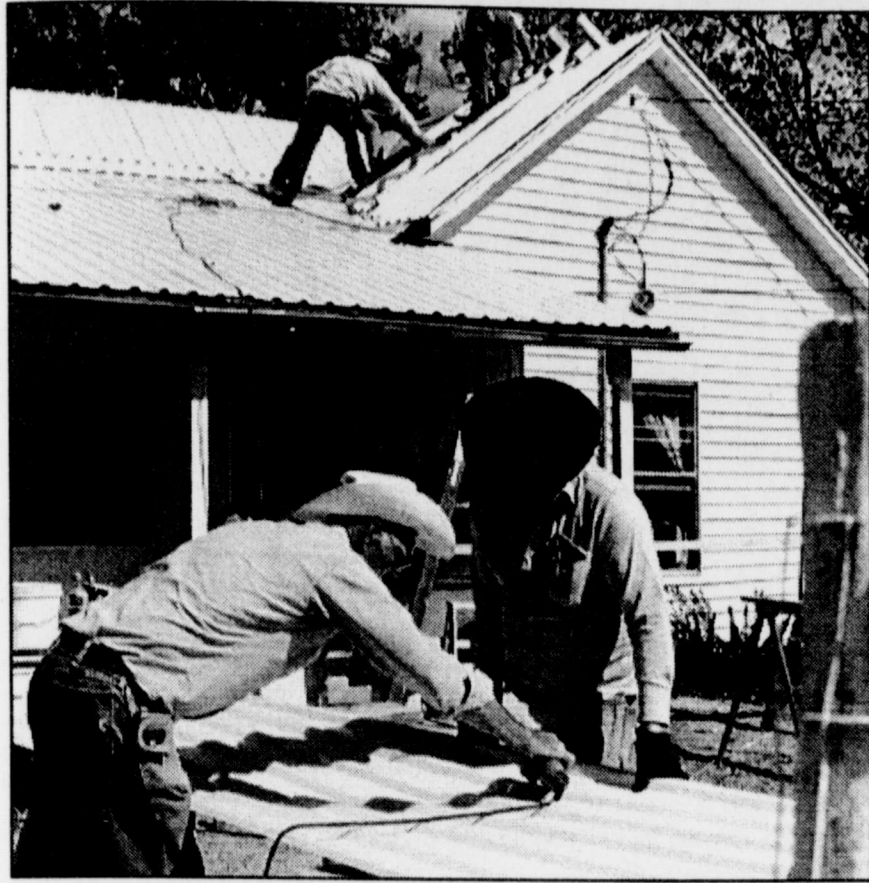
Garland O'Dell (left) and Billy Simpson cut metal to be sent to the roofing crew.
