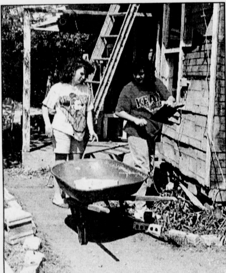
Adelaida Perez (left) and Diana Escalona fill another load of old siding while Michael Mostad does roof repair.
