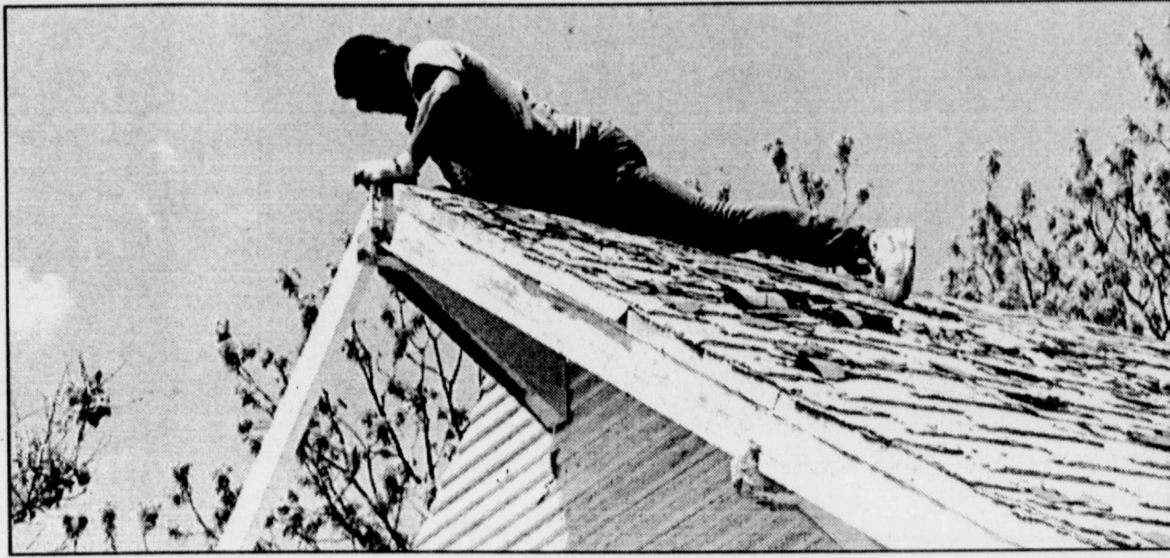
Robert Garza appeared to be king of the mountain as he perched precariously atop a roof being replaced.
