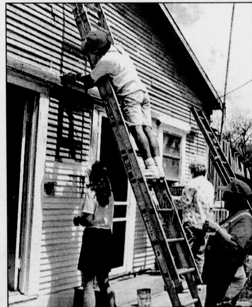
Cyndi Ashley and Pat Fenter paint from below while Alfonso Campos caulked above. Mary Ellen Moore enjoys a break from her inside painting job.
