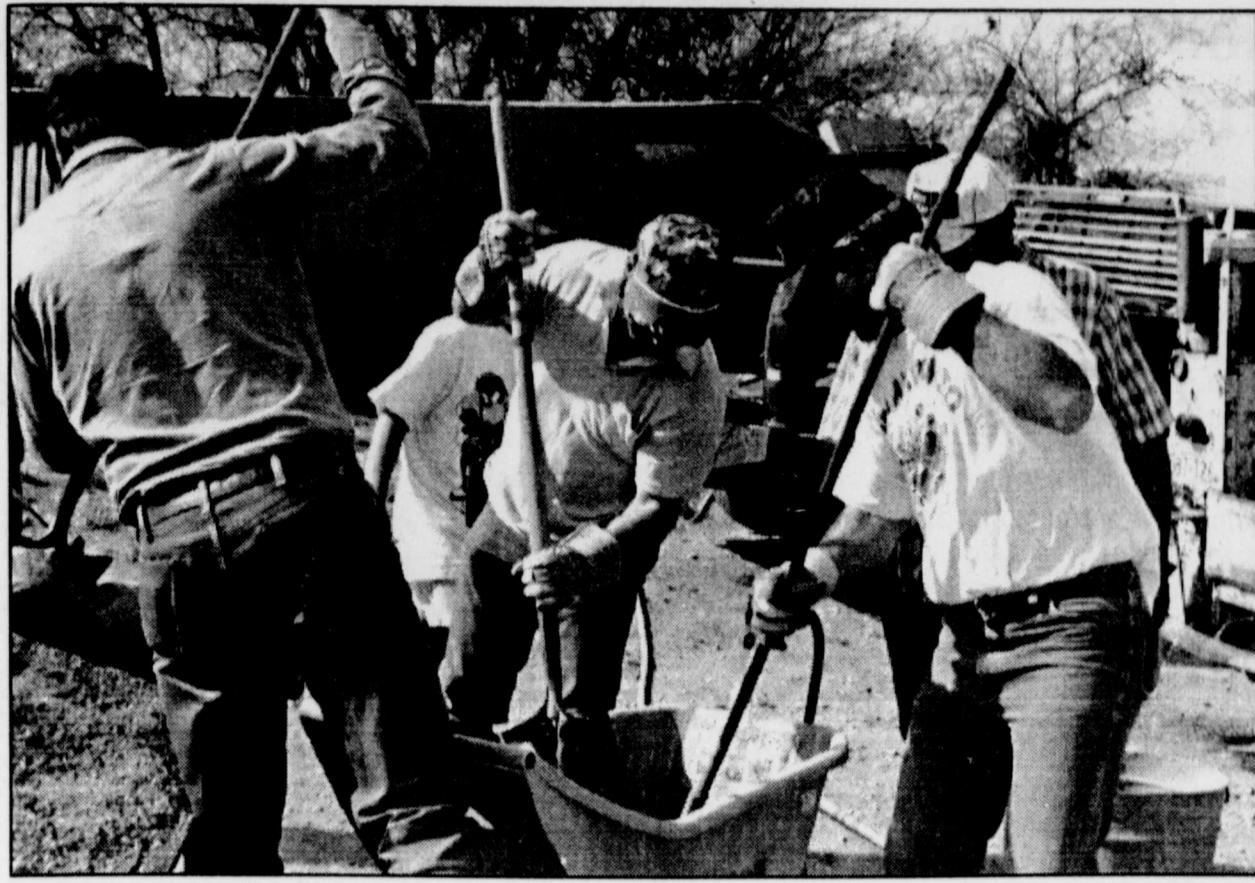
BUSY HELPERS (left to right) Brent Bryan, John Joeris, Darrell Kurtz, and John Parramore worked hard to mix cement for a new scoreboard to be placed at the Little League baseball field during the recent workday. Several men, women and children teamed together to prepare the fields for the upcoming season.
