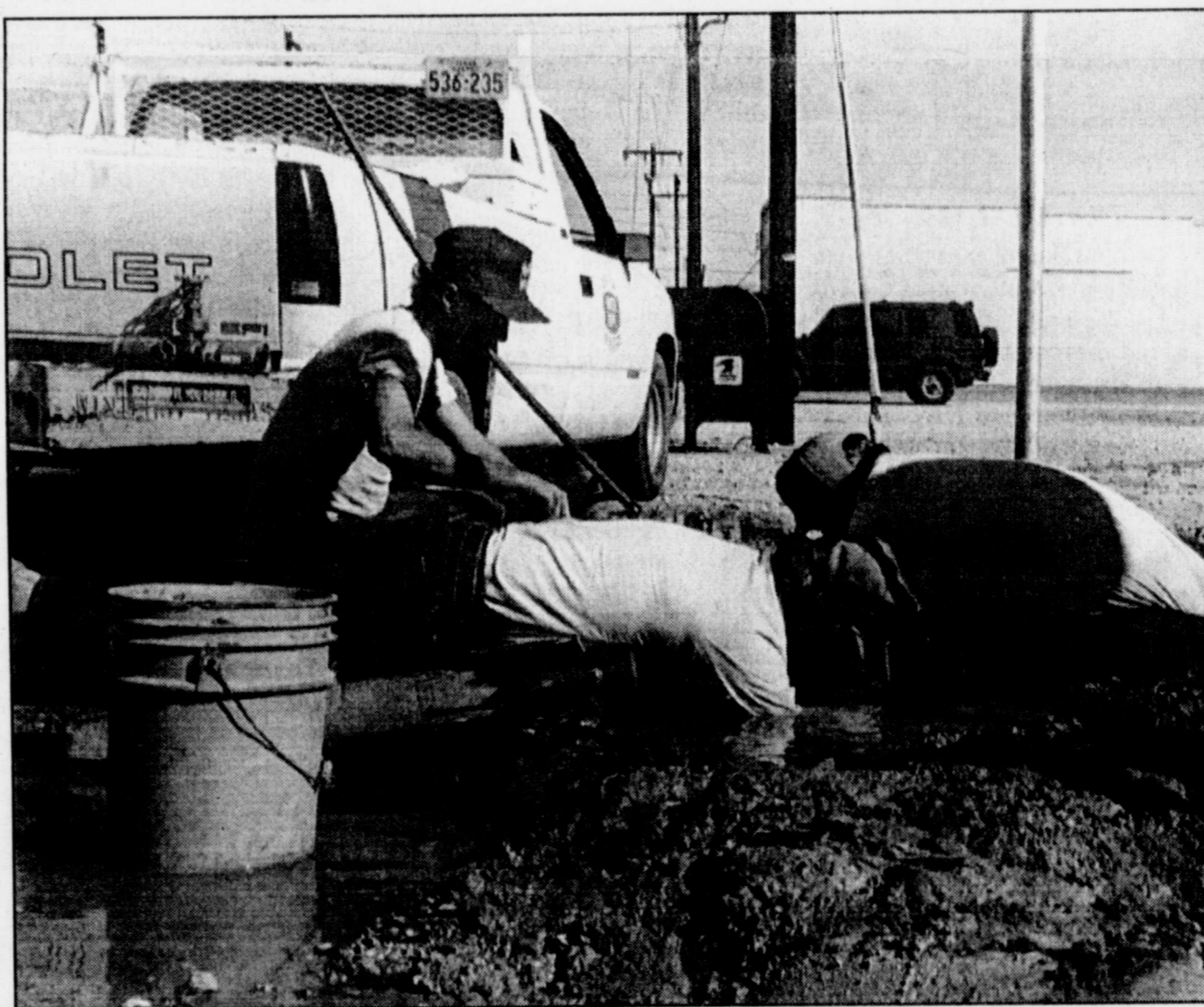
TAKING THE PLUNGE in 40 degree water were Street Department employees (left to right) Mike Scarborough, Tony Torres and Chuck Cravens, as they worked to repair a broken water main damaged by previous freezing temperatures.
