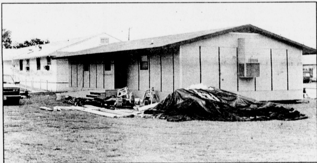
NEW HEADSTART CLASSROOM will soon be open at 601 W. Pierce upon completion of this 28'x52' building which will house one classroom, a kitchen, two bathrooms, storage area and office.
