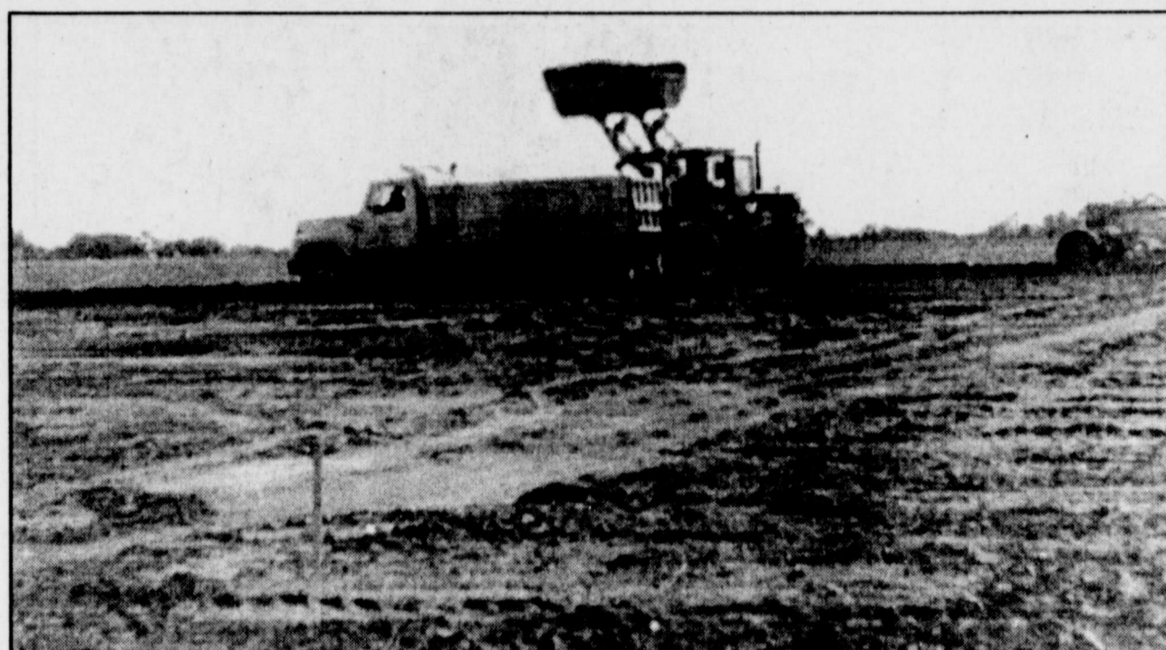
ABF TRUCKING has begun construction work for their new facility just north of town. The company hopes to finish the warehouse by the end of the year.
