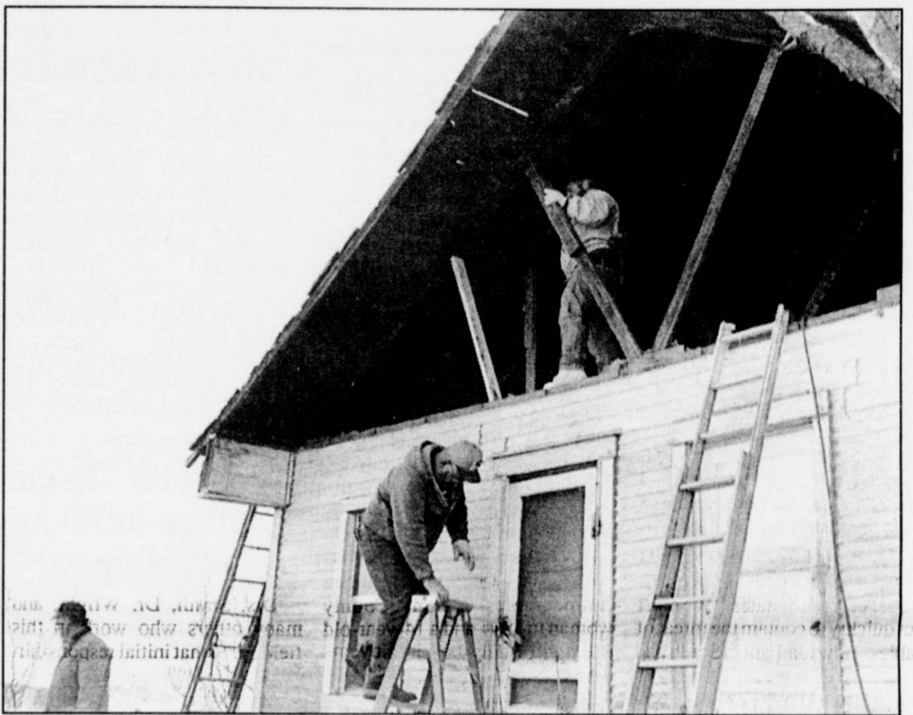
NEIGHBORS HELPING NEIGHBORS last Saturday as members of Christmas in April North Runnel, Inc. joined with members of the Norton Lions Club to renovate this home of an elderly Norton resident. Show at bottom left are Richard and Doyle Lange of Norton, Gary Moore on ladder and Jim Lincycomb in attic. Moore and Lincycomb are directors of Christmas in April of Winters.
