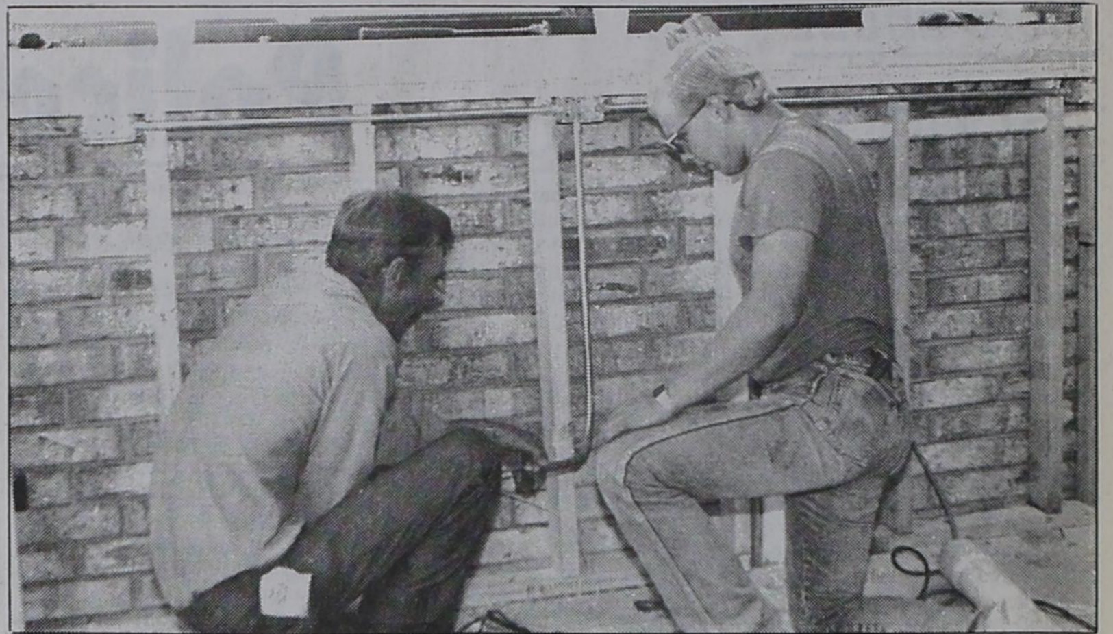
HART CLINIC BEING READIED—Electricians Dean Kirby (left) and Corey Mays install an outlet for a 220-volt circuit in the building that will house
