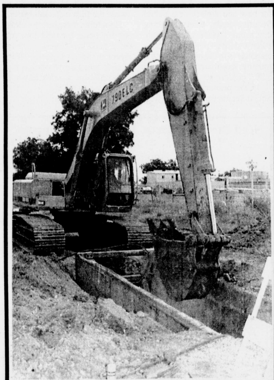
A PIPELINE WORKER with Roberts Construction Co. of San Angelo uses a John Deere excavator to dig out the sludge in the ditch being prepared for the new sewer line installed near Pioneer Vet Clinic on East Broadway by the City of Winters.
