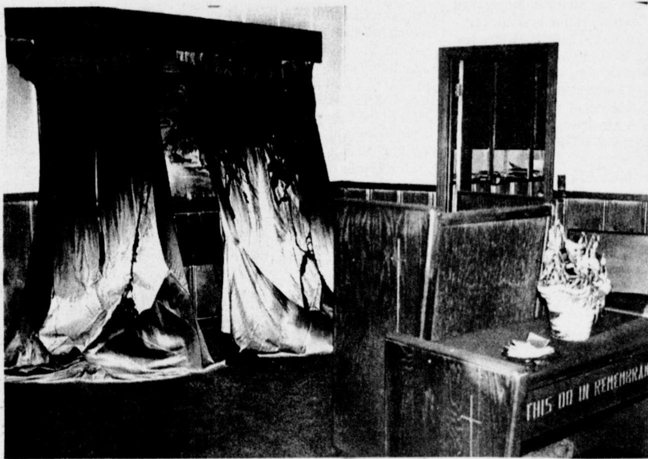
CHARRED AND MELTED remains of drapes, furniture and ceiling fans could be found inside Hopewell Baptist Church following Sunday night's fire.
