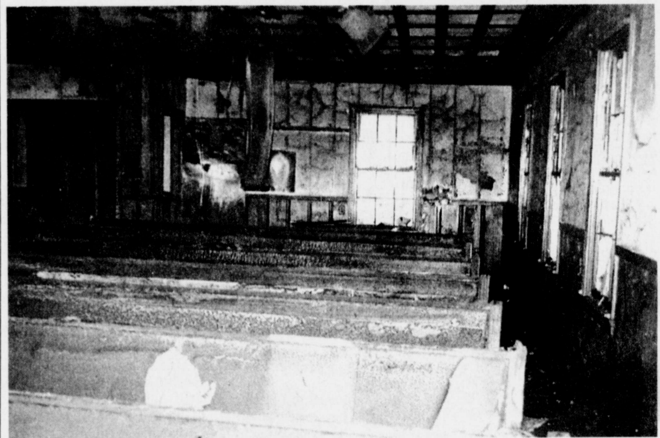
GUTTED INTERIOR showed extensive damage throughout. An official cause will be determined by a state fire marshal later this week.
