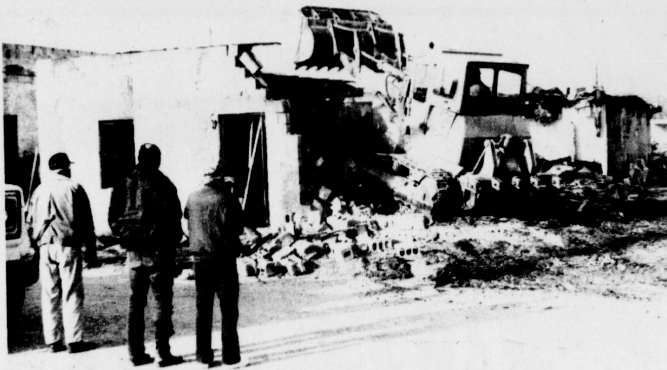
DOWN CAME THE OLD WALLS of the Midway Motel on Main street last week. The property was donated by Floyd and Halley Sims to the volunteer fire department as the site of a new fire station to be built within the next year or so. The new facility will have a training room, an office and eight bays for fire equipment.
