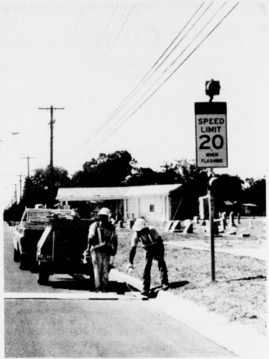
SIGNALS INSTALLED—Last week workers from the Texas Department of Transportation installed school zone signal lights and speed limit signs on Main Street and on Novice Road.
