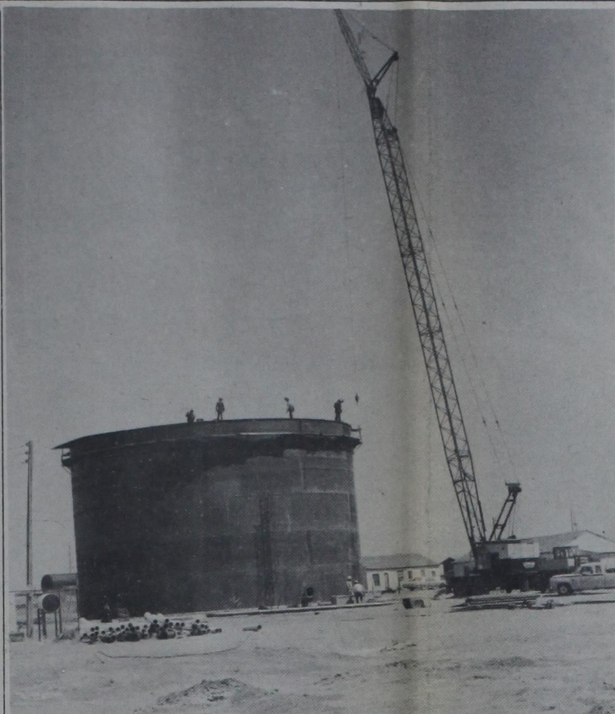
GOING UP - Construction of the city's million gallon water reservoir in Southeast Dimmitt continued last week as workmen were busy welding on the upper level of the huge metal storage tank. Upon completion the facility will give the city's water system a needed boost.
